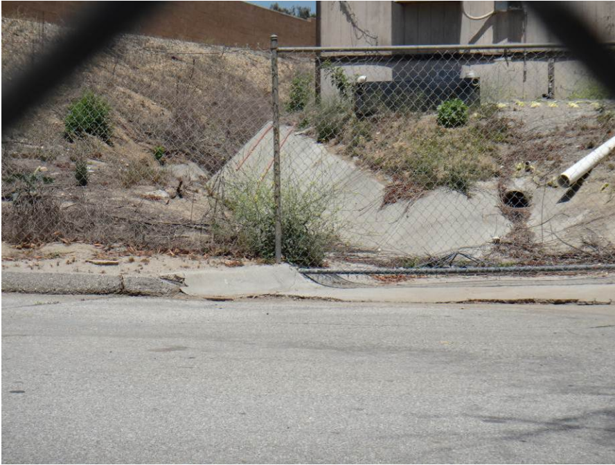
Photograph 25: Upstream portion of ephemeral drainage Feature 7-38-S-1, taken from west side of Greenwood Road, facing upstream/east.
