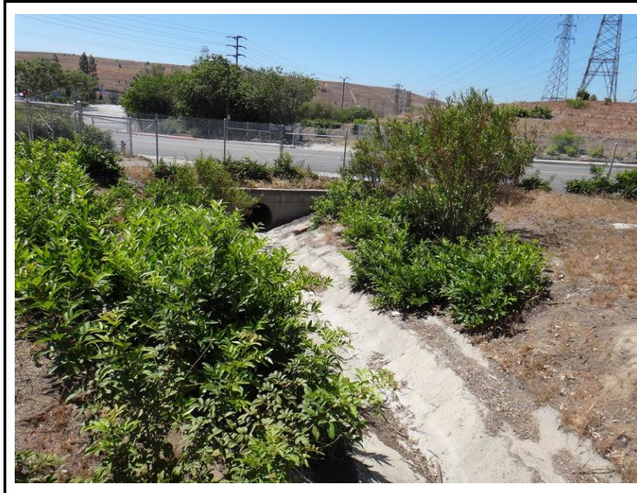
Photograph 27: Ephemeral drainage Feature 11-136-S-100, facing downstream/south.
