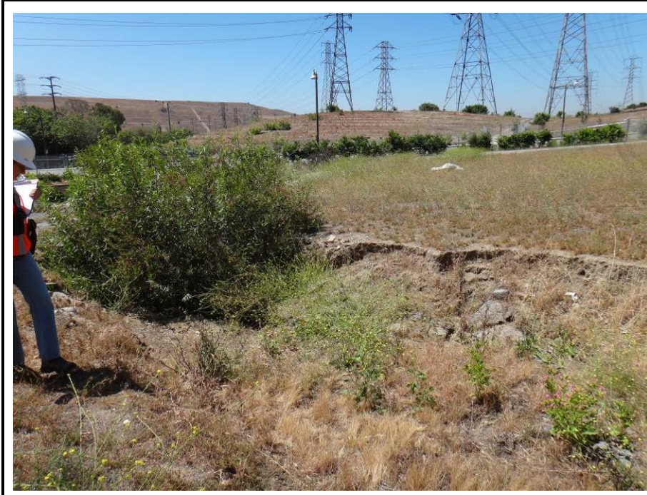
Photograph 29: Northern dirt-lined portion of ephemeral drainage Feature 11-136- S-100, facing downstream/south.
