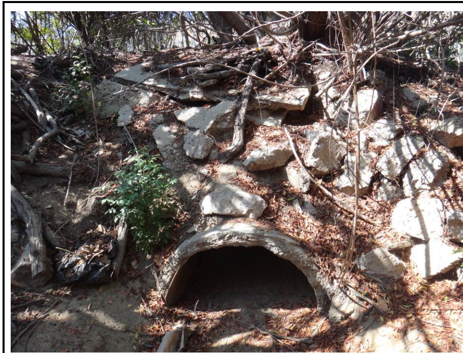
Photograph 23: Culvert at the upstream portion of ephemeral drainage Feature 11-136- S-101, facing north.
