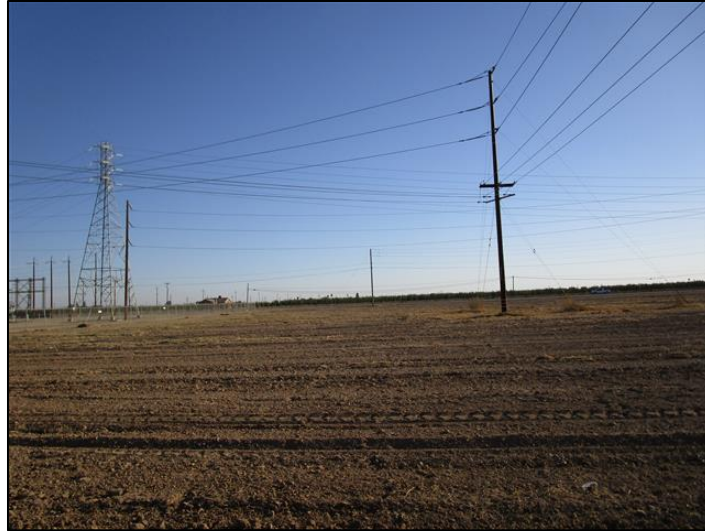
Photo 4. View facing south, northwest of Sanger Substation within the temporary staging area. 36.709022, -119.612176.
