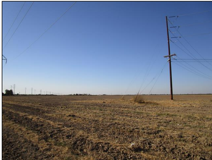
Photo 1. View facing northwest of Sanger Substation from E. Jensen Avenue. 36.706697, -119.612205.
