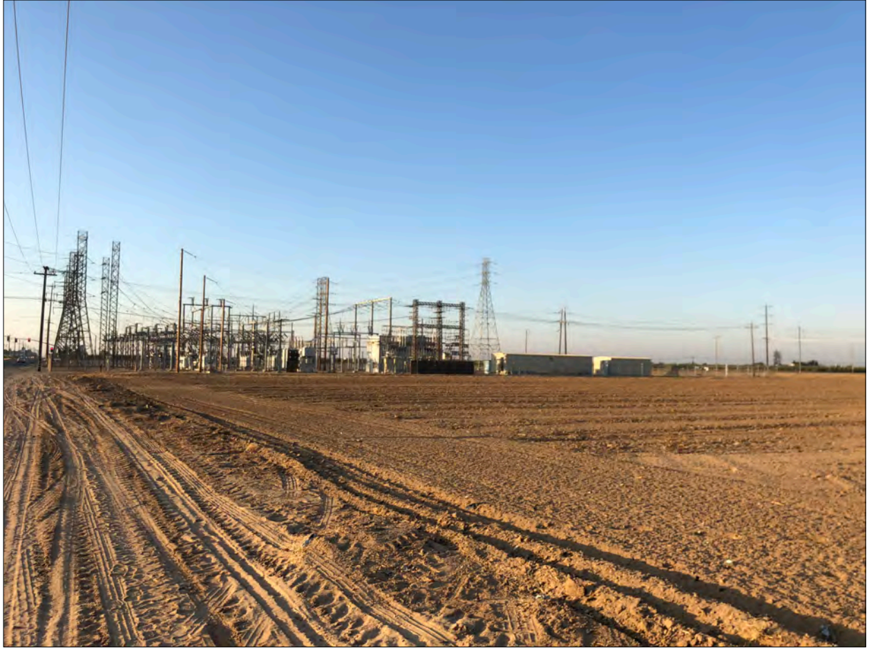
Figure 4. Photograph of the expansion footprint, looking south, showing a recently disked field.
