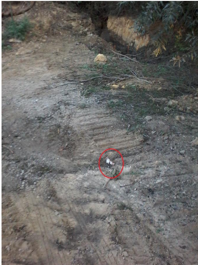
Photo 10: ESA flagging and a stake knocked over and underneath bulldozer tracks within the Rincon Creek ESA buffer along Segment 3B. November 21, 2017 (Photo by SCE)
