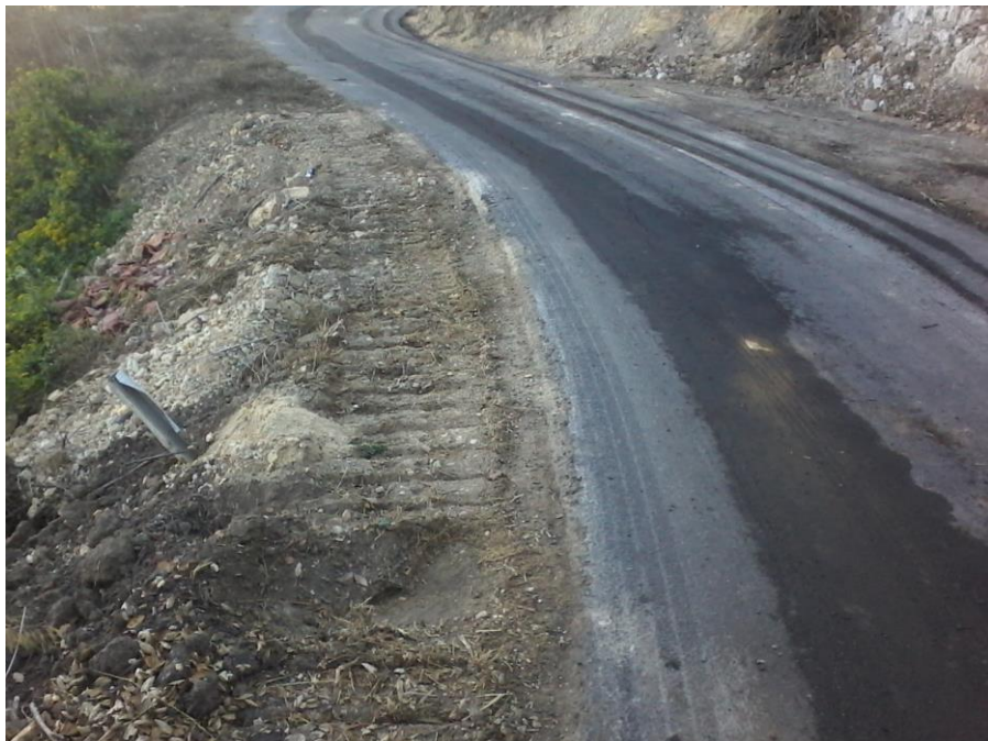
Photo 8: Bulldozer tracks outside of disturbance limits within the Rincon Creek ESA along Segment 3B. November 21, 2017 (Photo by SCE)
