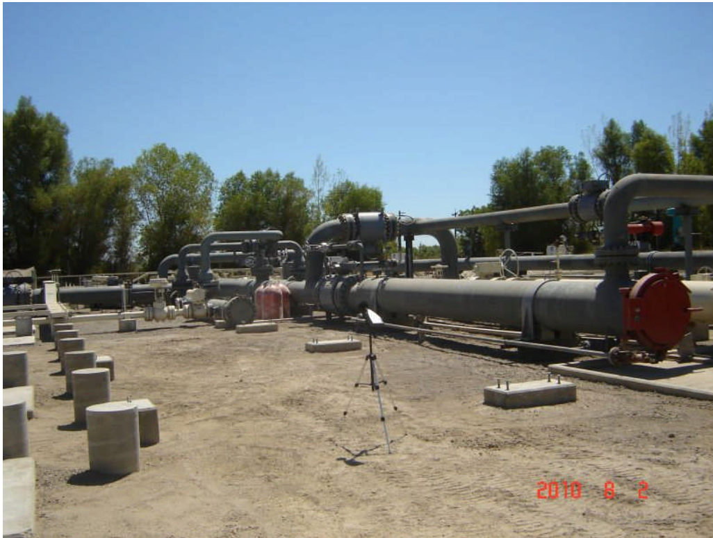
Figure B-1. Site 1 (50 Feet from Center of Equipment at WPS)
