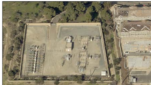
San Ysidro Substation (Pictometry.com 12/24/2014)
