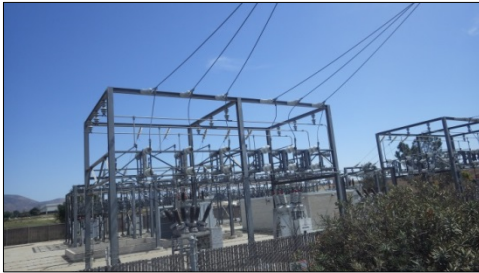
Border Substation (HDR 3/22/2015)
