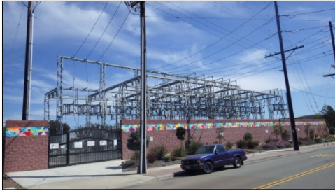
Otay Substation (HDR 3/22/2015)
