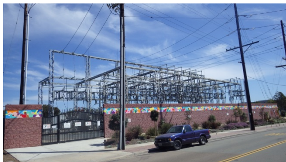
Otay Substation, looking southeast. March 23, 2015
