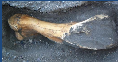
A mammoth femur, approximately 3 feet long, found while excavating a pipeline trench.
