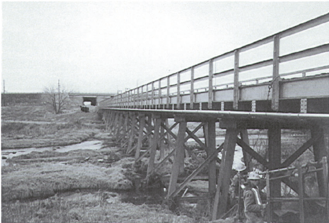
Cables are in pipe attached to side of bridge.
