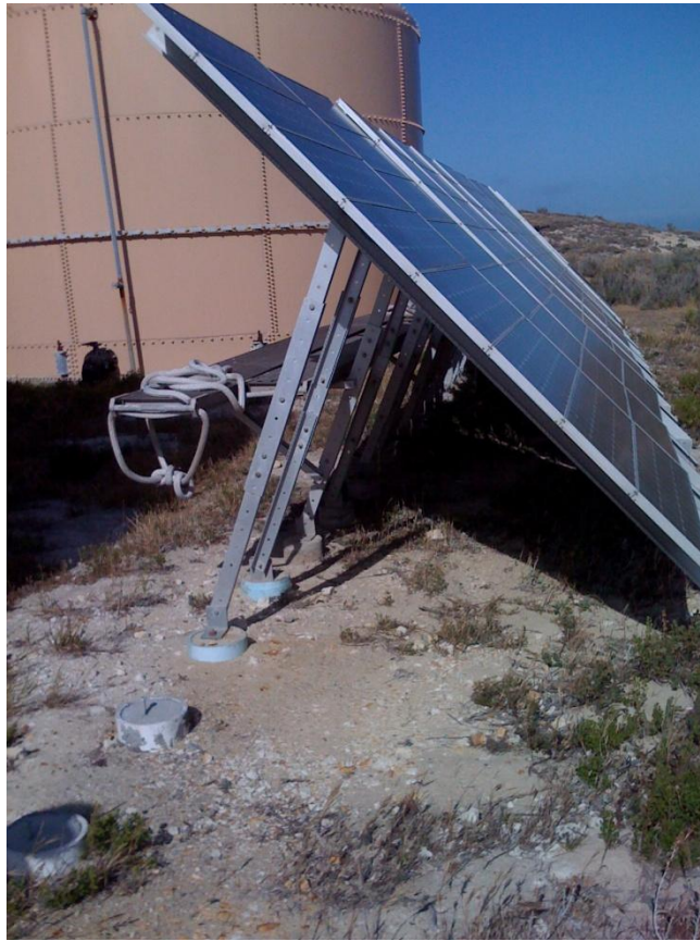
Figure 1 – Clarification on Solar panel at Santa Rosa Maintenance Area
