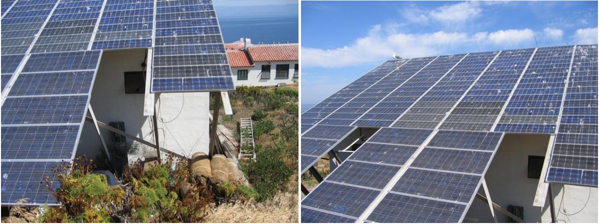
Figure 21 – Anacapa Solar Panels at Solar Building Lat 34° 00'54.60" N, Long 119° 21' 48.45" W
