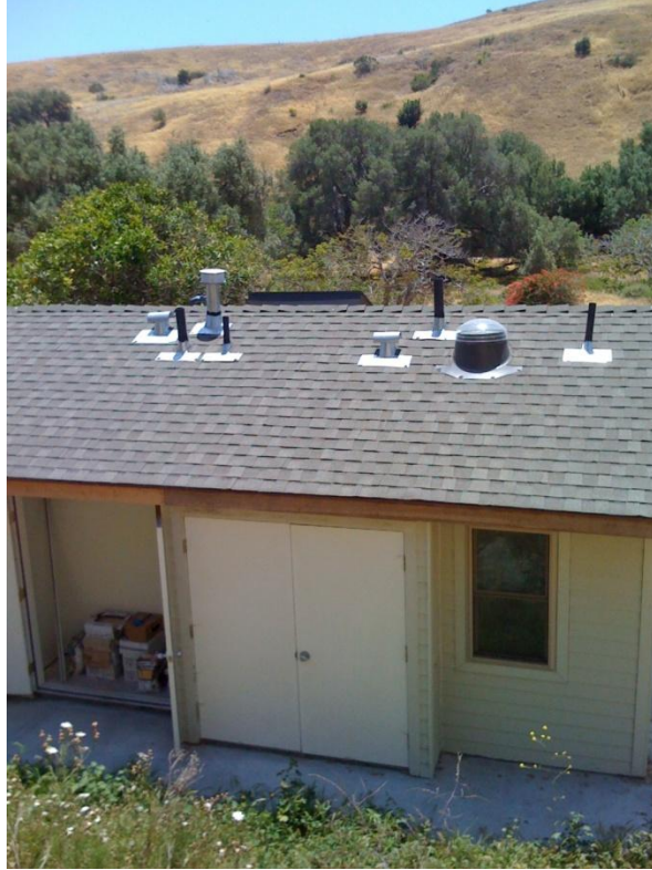
Figure 5 –Back wall of the Smugglers Bathroom building
