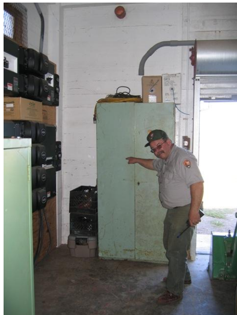
Figure 23 – Anacapa inside location for equipment
