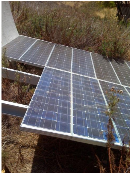
Figure 3 – Solar Panel behind Smugglers bathroom Building
