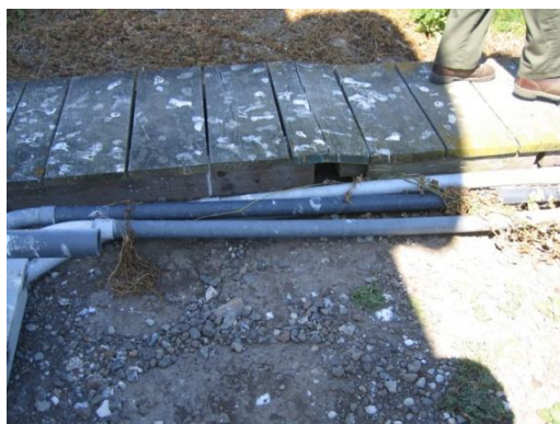
Figure 27 – some existing conduit between solar panels and Generator Building on Anacapa
