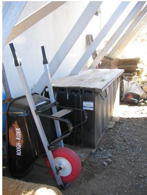
Figure 24 – Anacapa Battery Bank Outside
