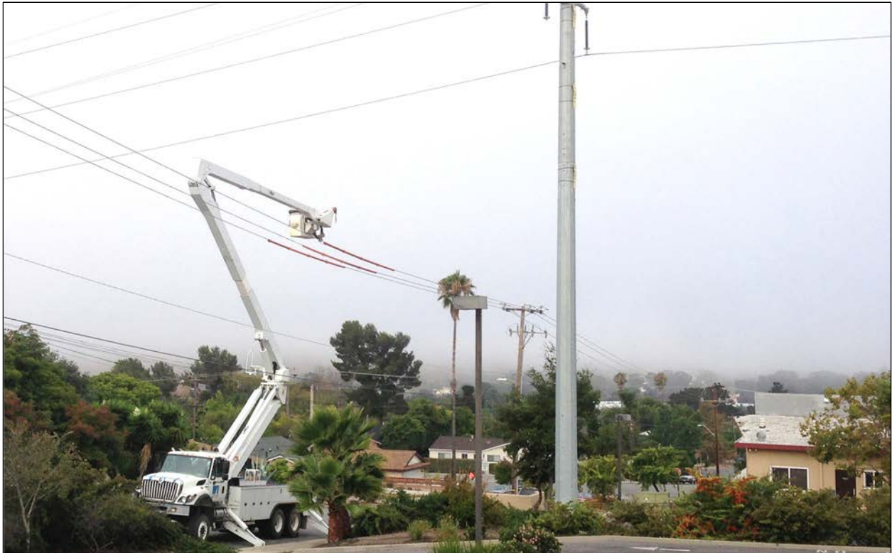
Figure 2.6-4 Positioned Equipment Guard Structure
