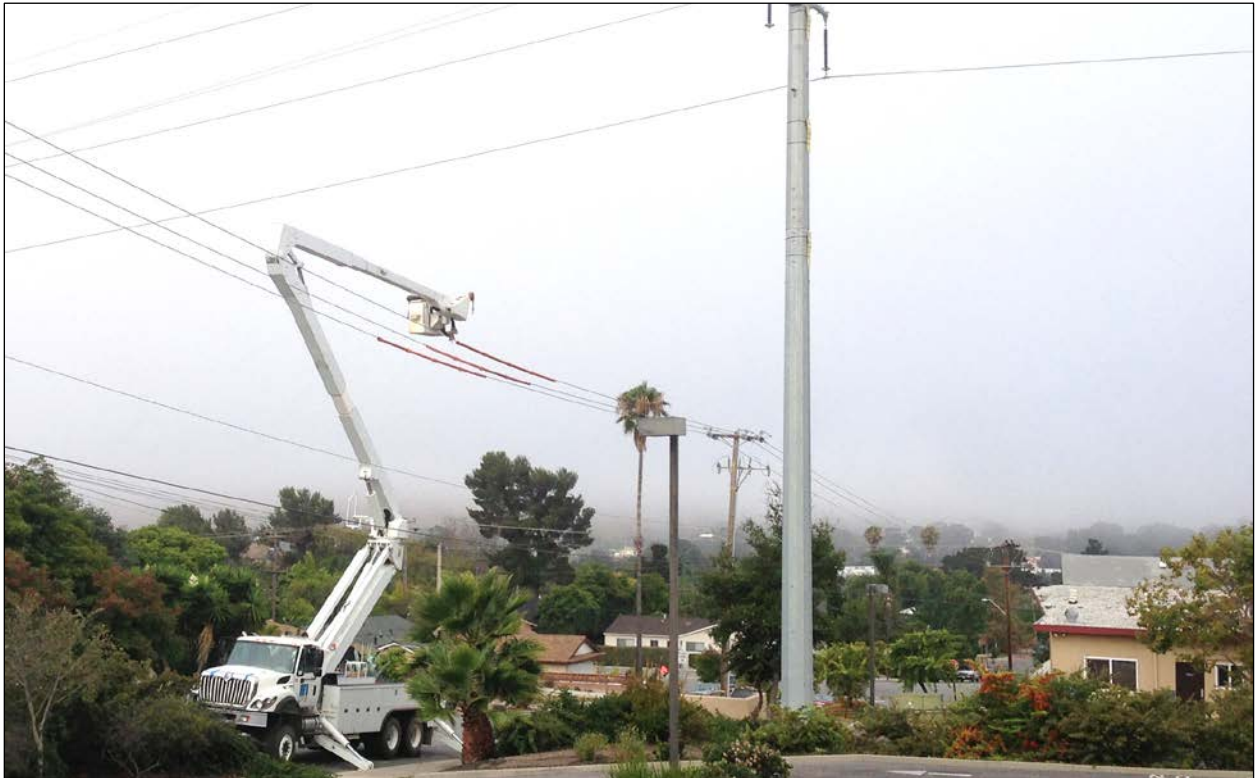
Figure 2.6-4 Positioned Equipment Guard Structure
