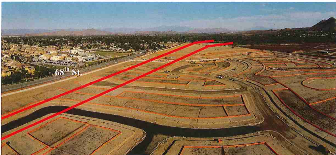
Photo 2: Looking east with 68 th Street on the left. The picture show walls under construction and streets ready for asphalt. [The RTRP proposed easement is shown in red (approximate)]
