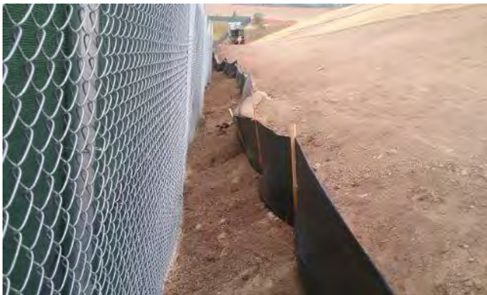
Caption Potentially weak area in erosion control fencing.
