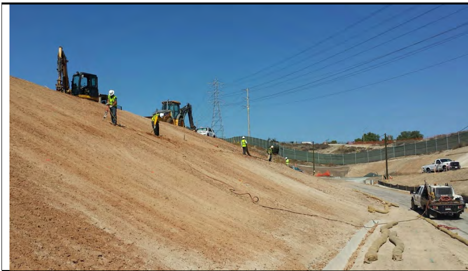
Photograph 4: Installation of straw wattle BMPs along the slope of the substation pad during the week of October 15, 2016.
