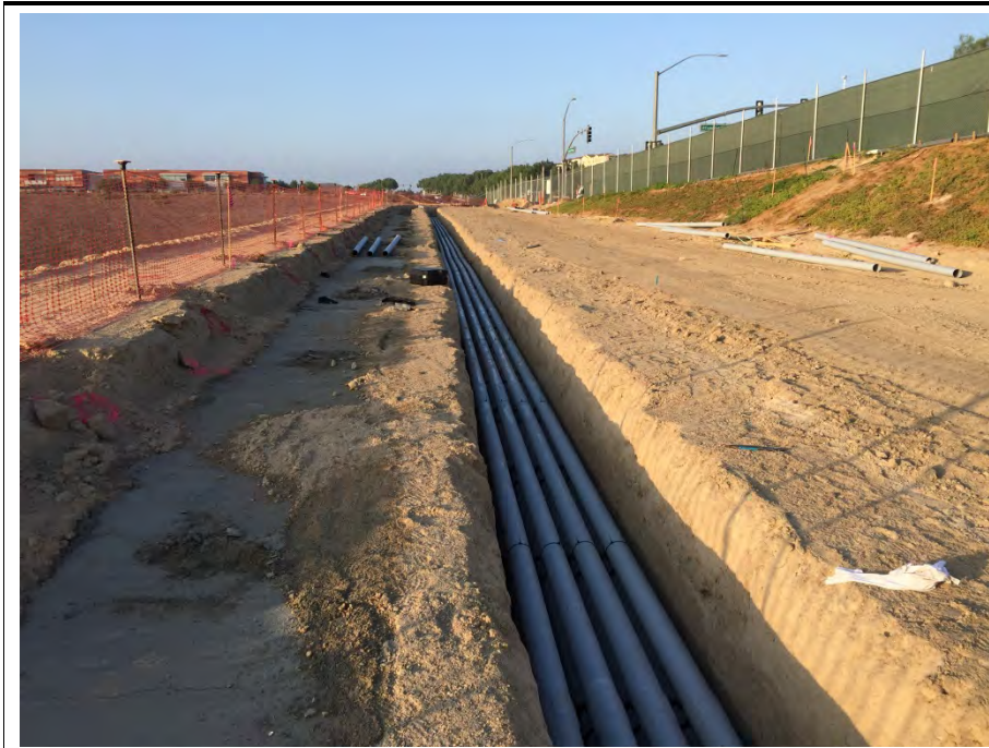
Photograph 2: Installation of PVC conduit for the 12kv getaway occurred during the week of October 24, 2016.
