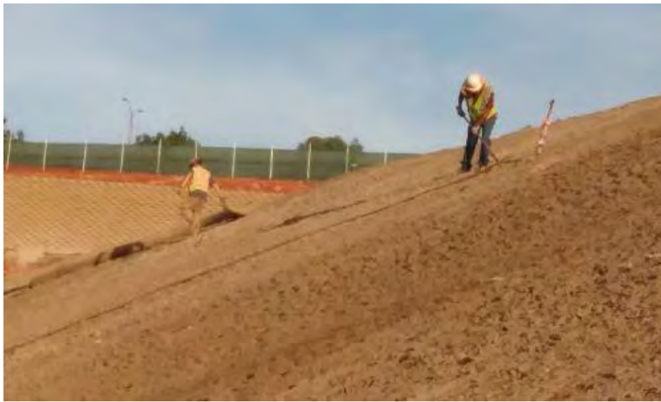
Caption Straw wattle installation on finished slopes on west side of site.
