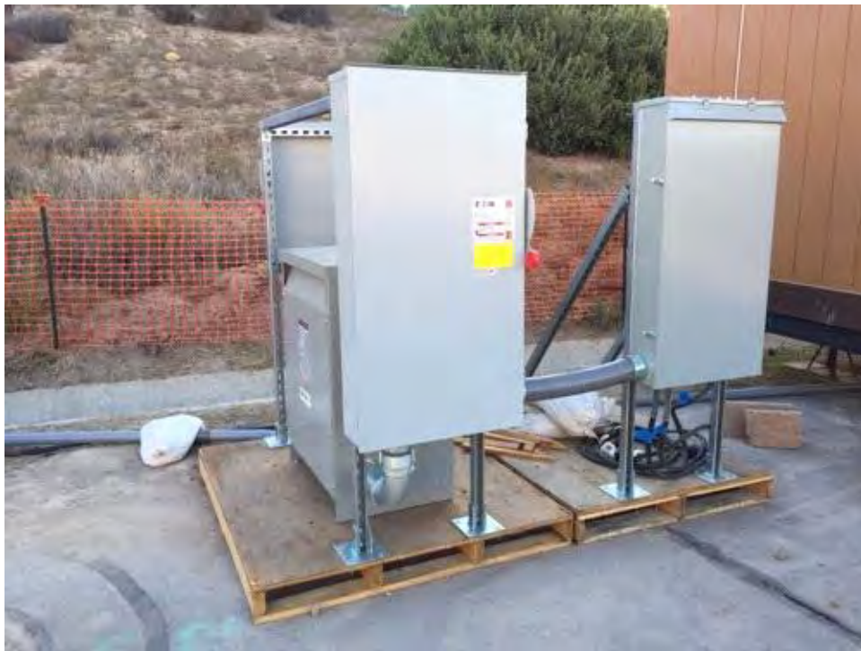
Caption Disconnect and circuit panels.
