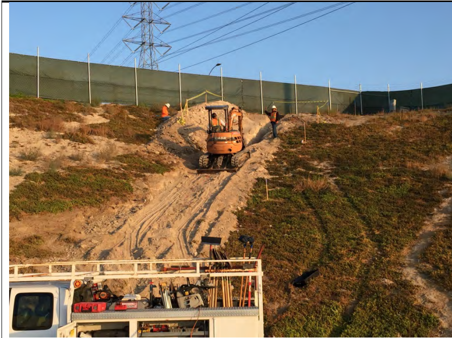
Photograph 1: Excavation of trench for water lines occurred during the week of October 24, 2016.
