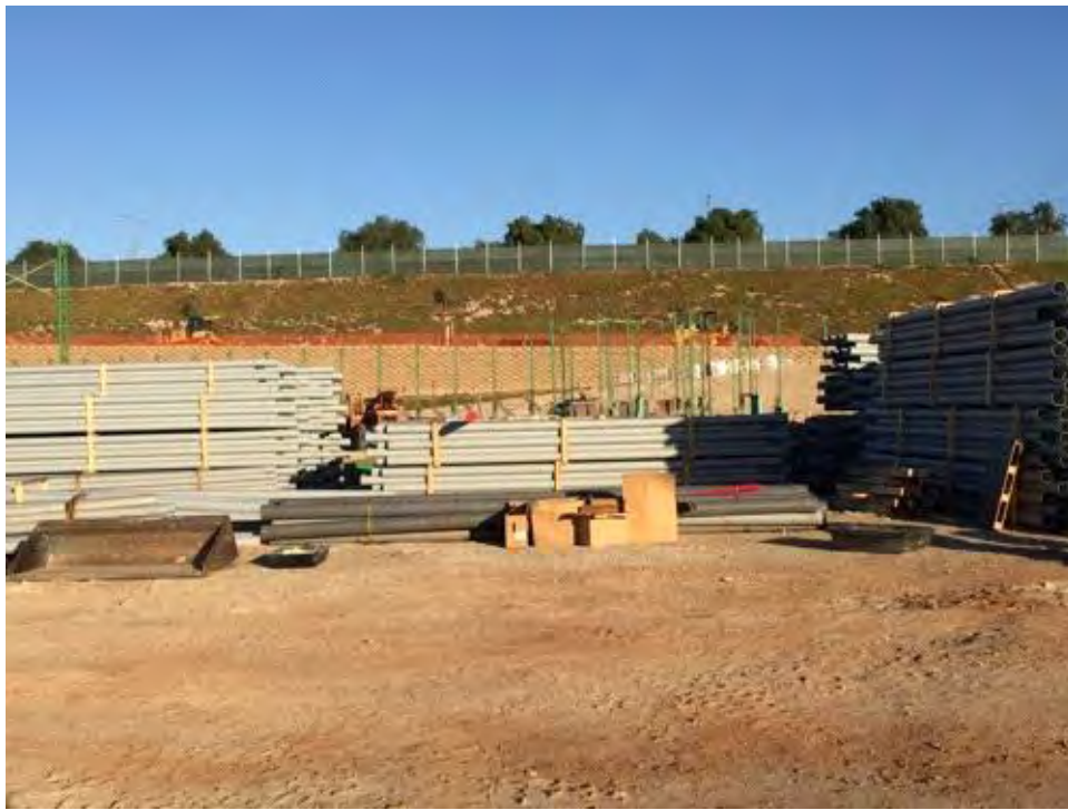
Caption Conduit pipe for 12 kv line.
