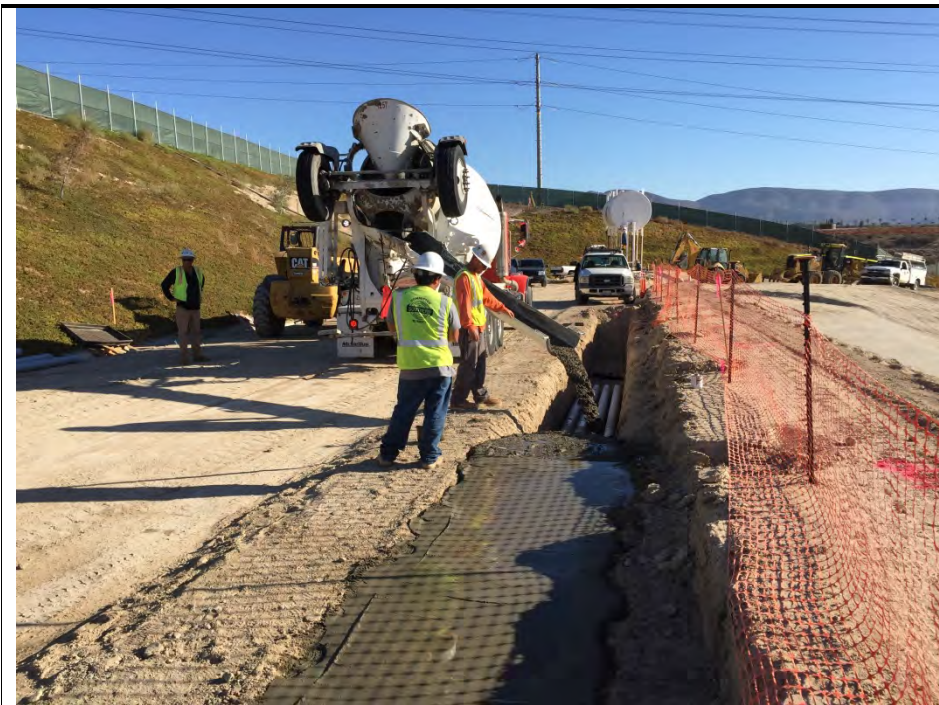
Photograph 4: Numerous slurry pours over 12KV conduit (distribution lines) occurred during the week of October 17, 2016.
