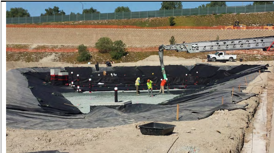
Photograph 2: Installation of the bio-retention pond base material during the week of October 15, 2016.
