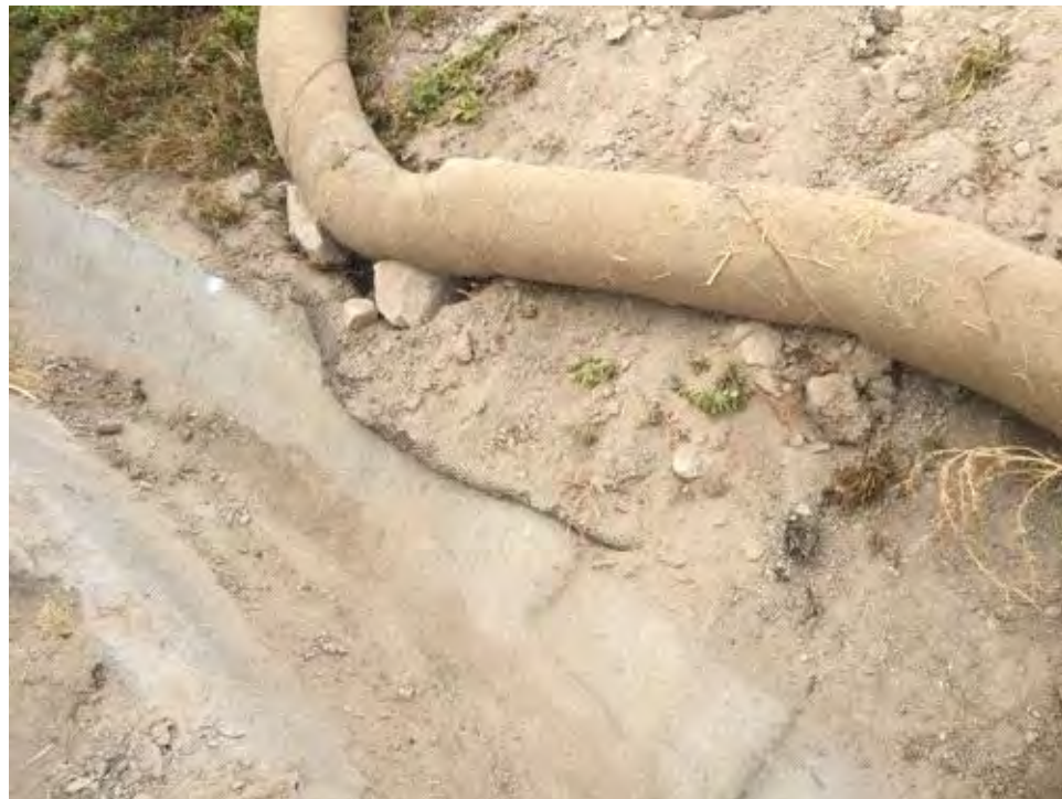
Caption Repair needed above brow ditch along north access road.
