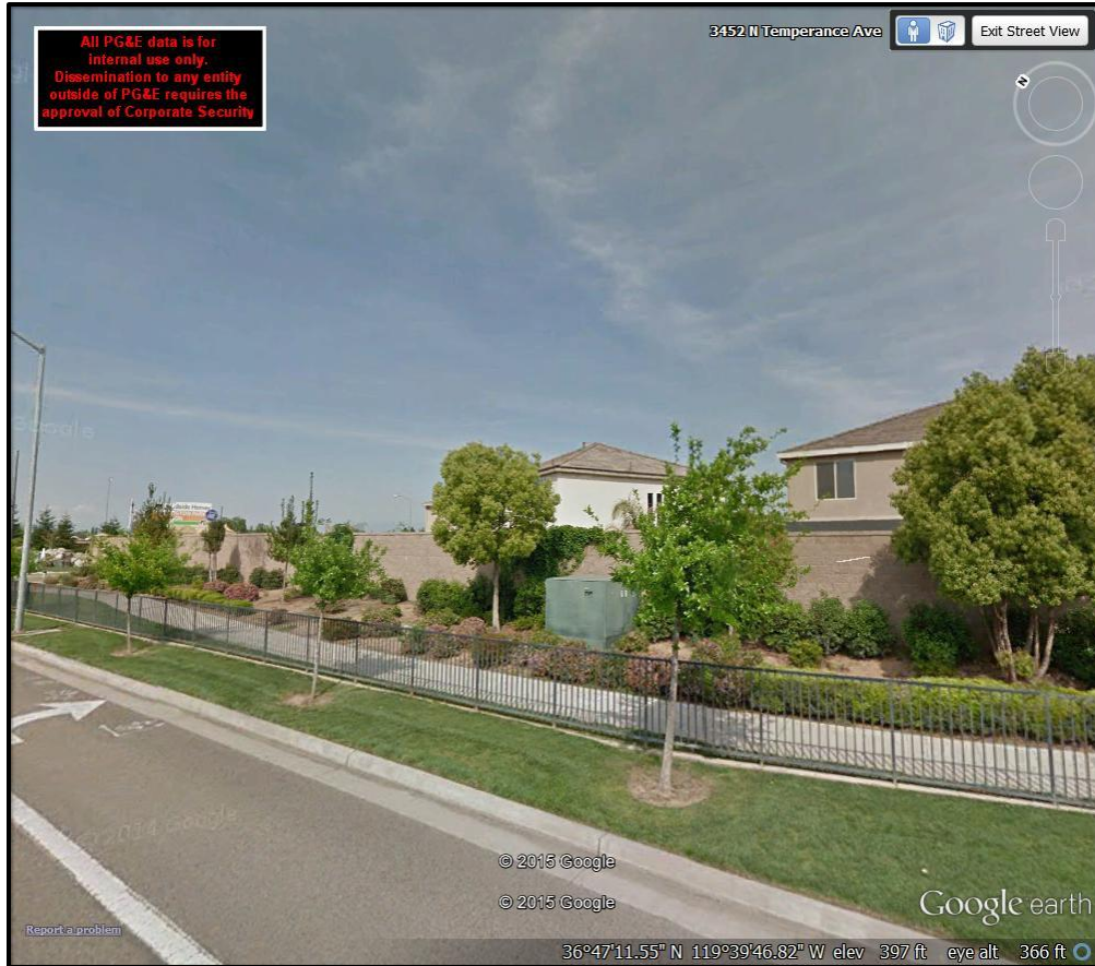
Figure 5. Representative image of capacitor bank.
