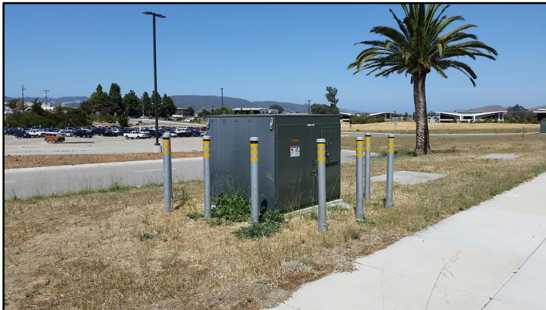
Figure 4. Representative image of capacitor bank.
