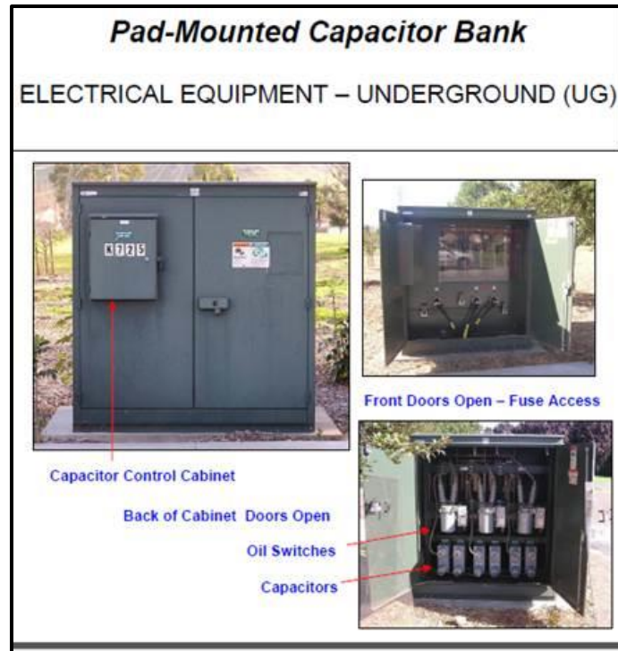
Figure 3. Representative image of capacitor bank without barrier posts.
