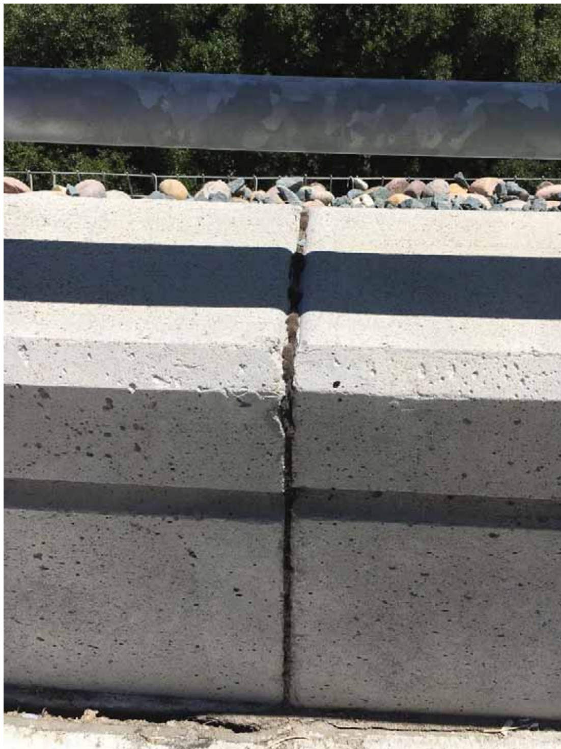
Photo 9: Pavement differential settlement
