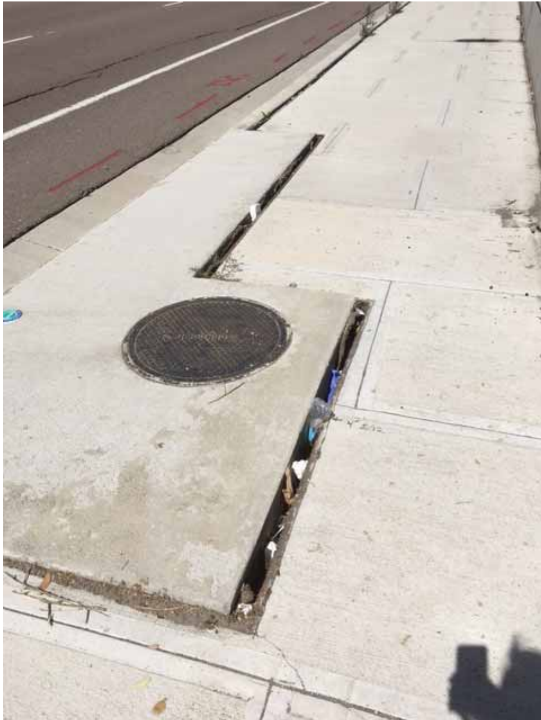
Photo 8: Pavement differential settlement
