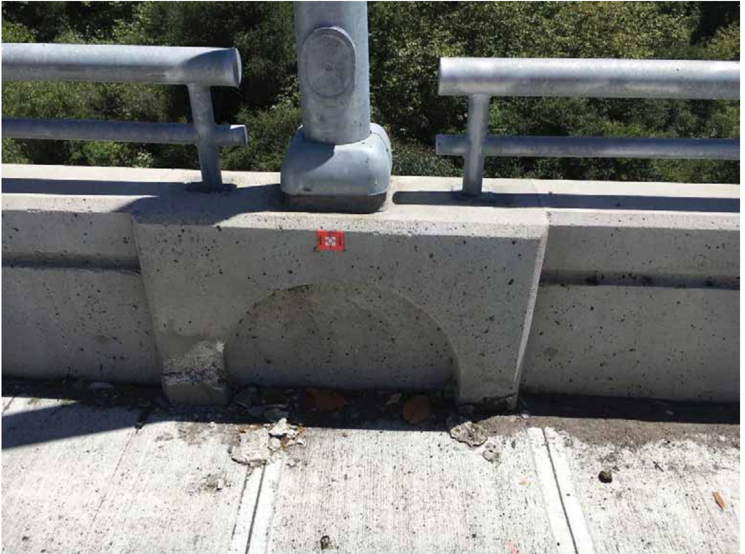
Photo 14: Pavement differential settlement
