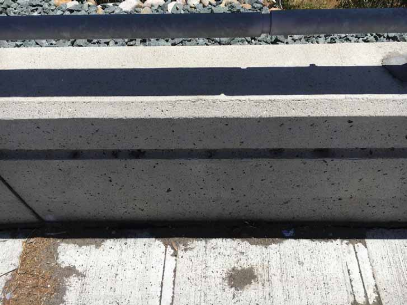
Photo 12: Pavement differential settlement
