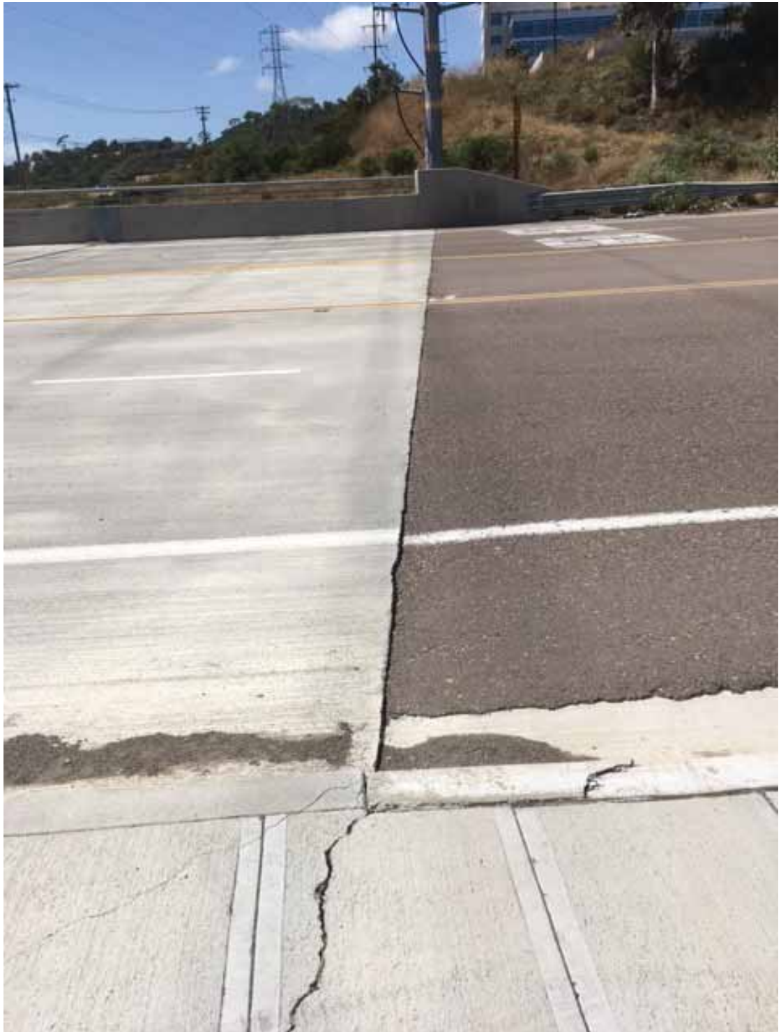
Photo 6: Pavement differential settlement
