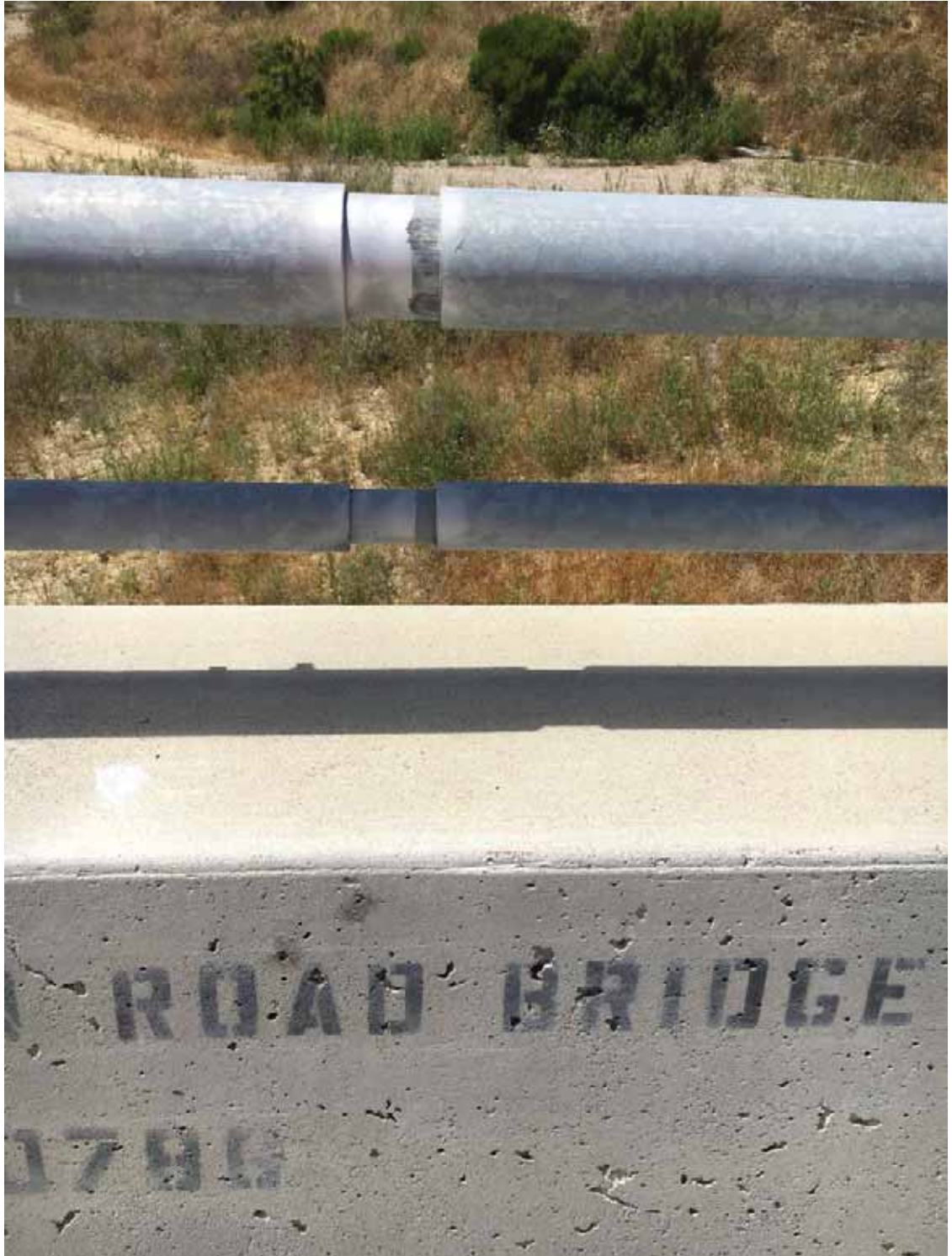
Photo 16: Pavement differential settlement
