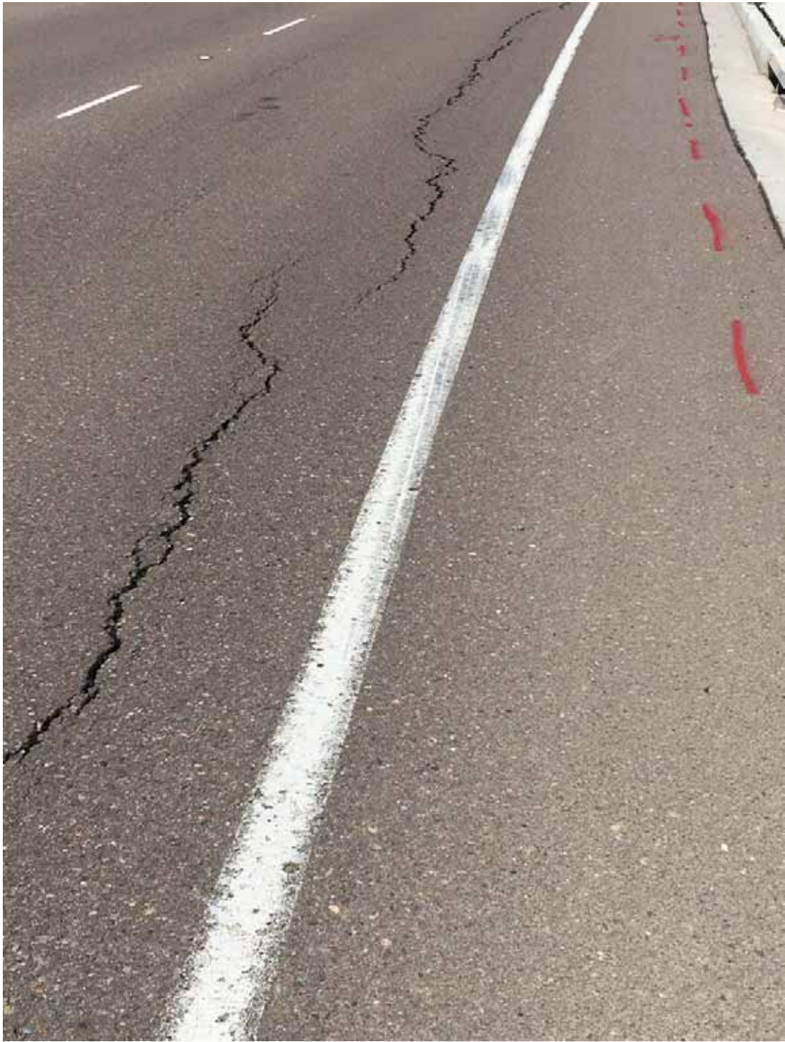
Photo 1: Pavement differential settlement
