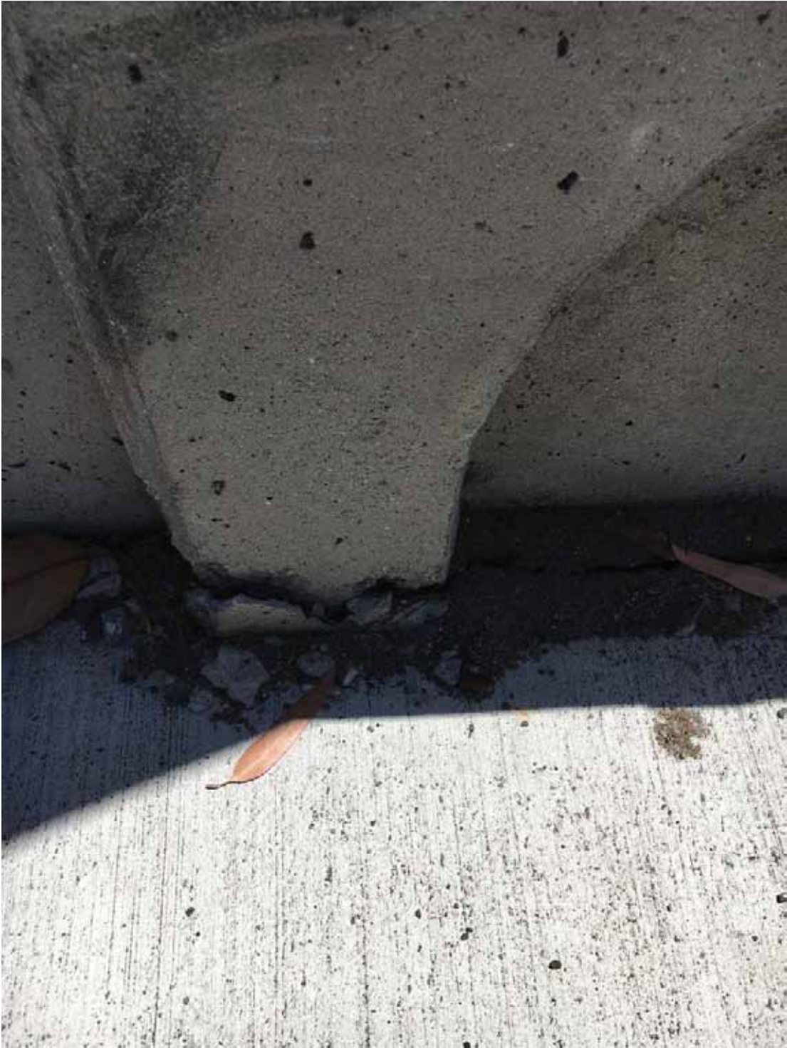
Photo 11: Pavement differential settlement
