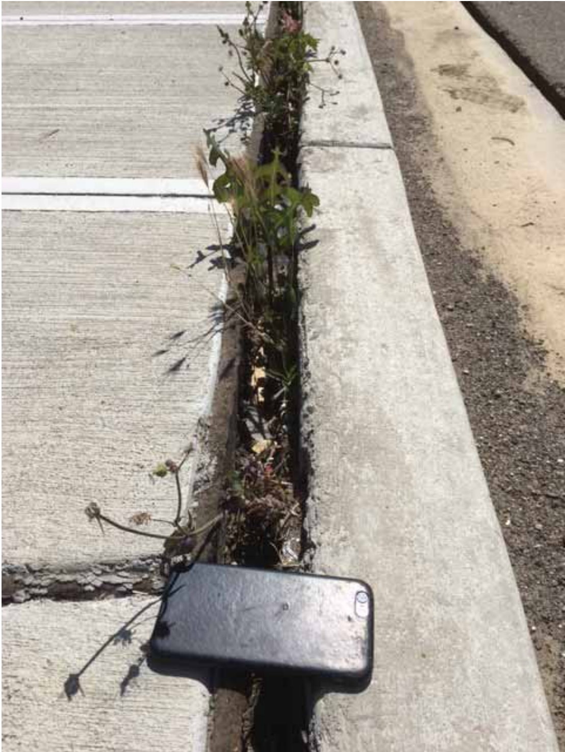
Photo 5: Pavement differential settlement
