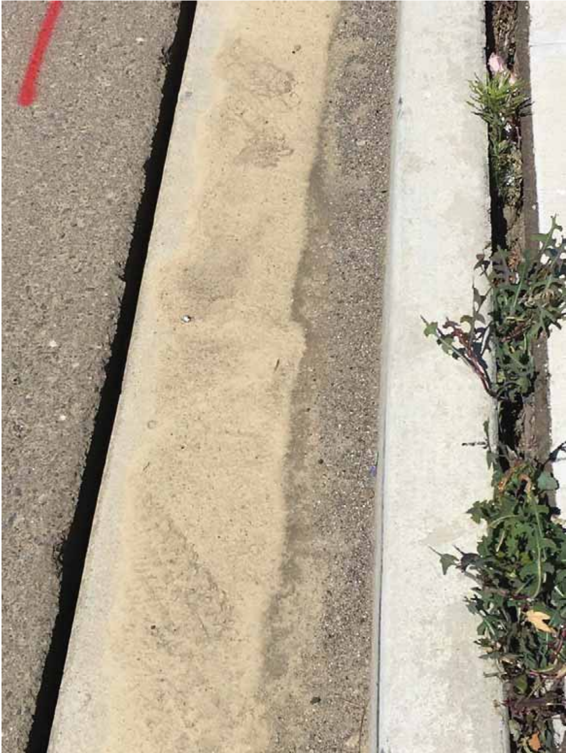
Photo 3: Pavement differential settlement
