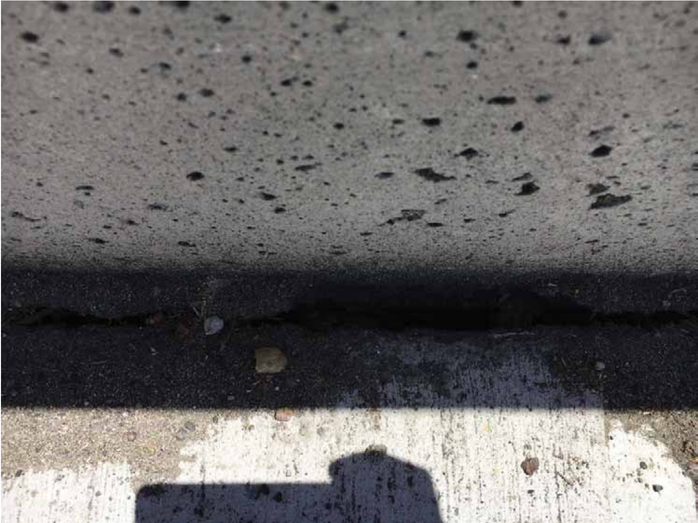
Photo 13: Pavement differential settlement
