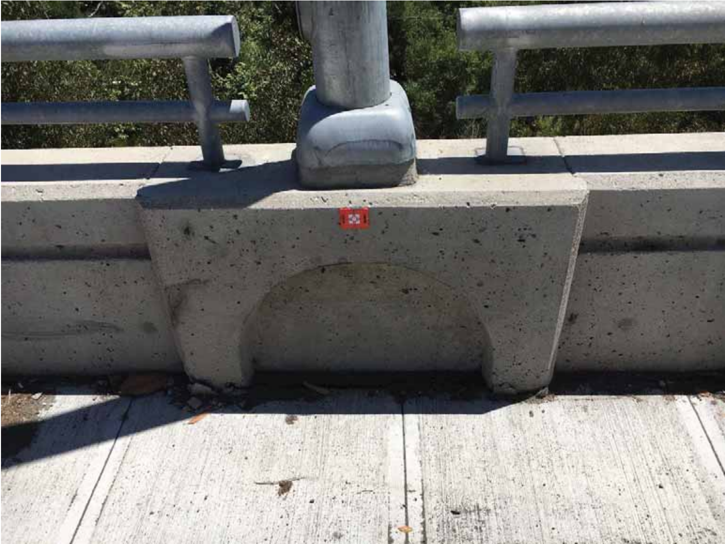
Photo 10: Pavement differential settlement
