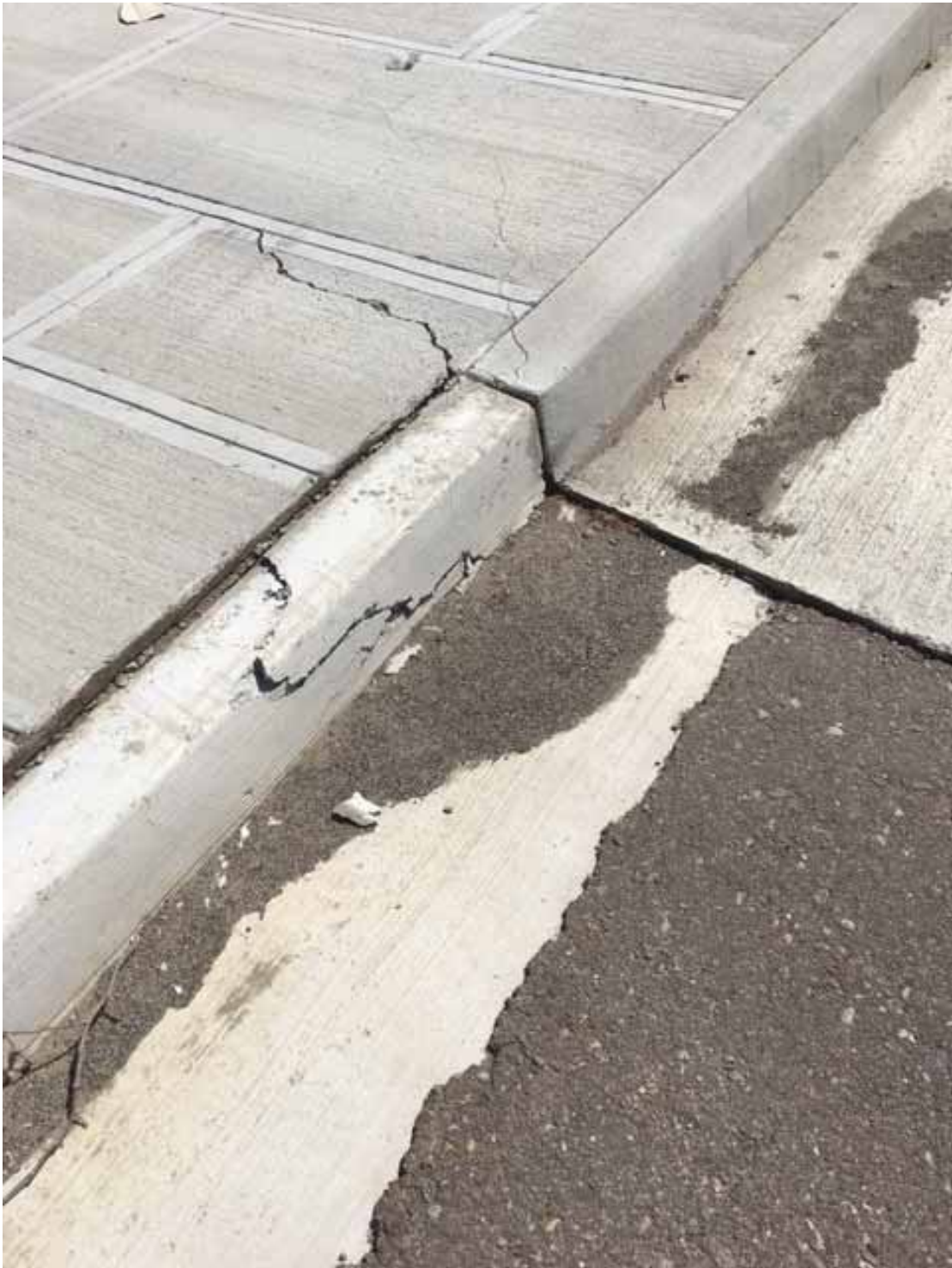
Photo 7: Pavement differential settlement
