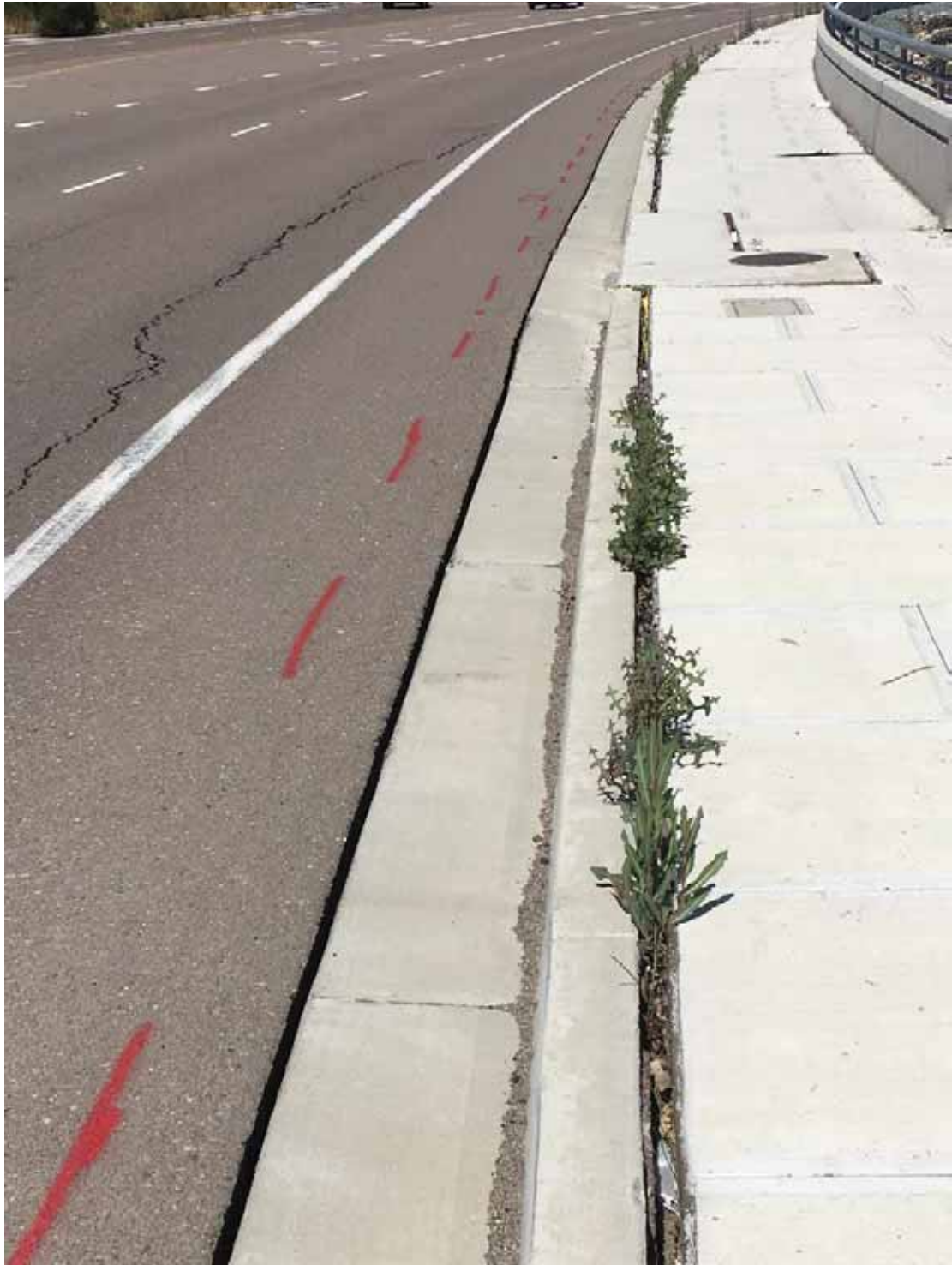
Photo 2: Pavement differential settlement
