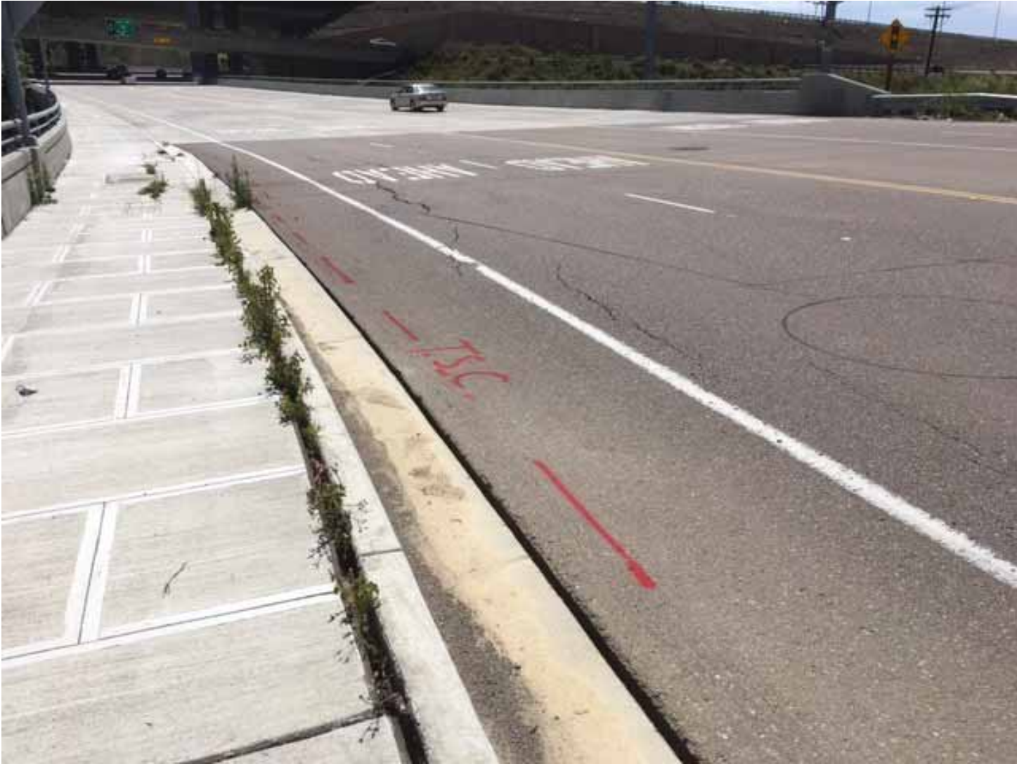
Photo 4: Pavement differential settlement
