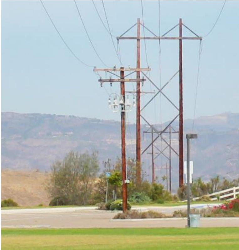
Figure 2.3-7: Typical Topped H-Frame Structure
