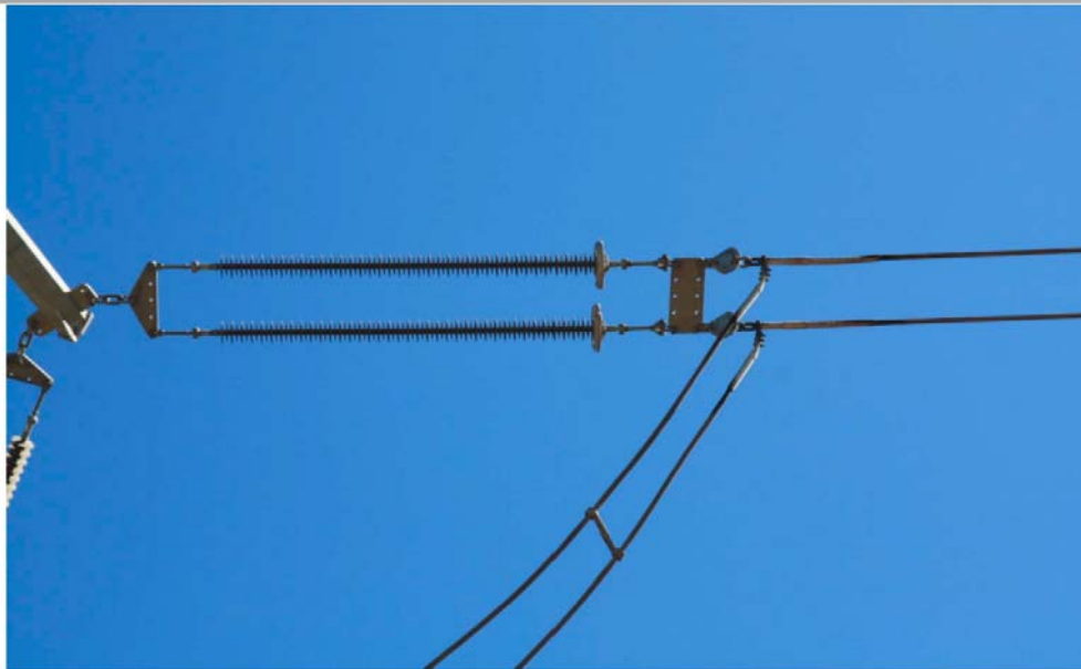
Figure 2.3-3: Representative Photograph of Bundled Conductor
