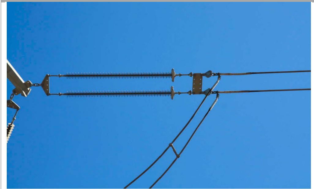
Figure 2.3-3: Representative Photograph of Bundled Conductor
