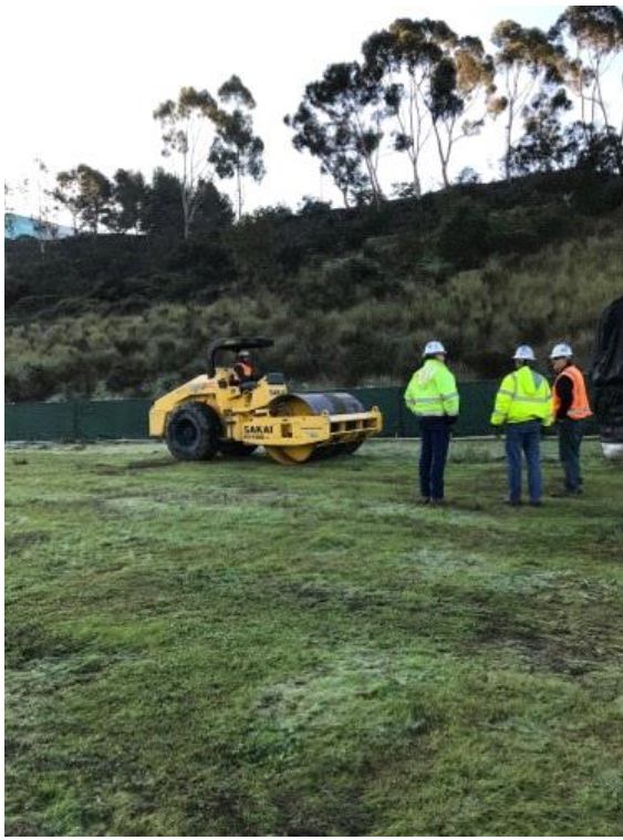
Caption Rolling site in preparation for laying ground rock at Driving Range Yard.
