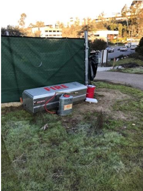
Caption Firebox and spill kit at Driving Range Yard.
