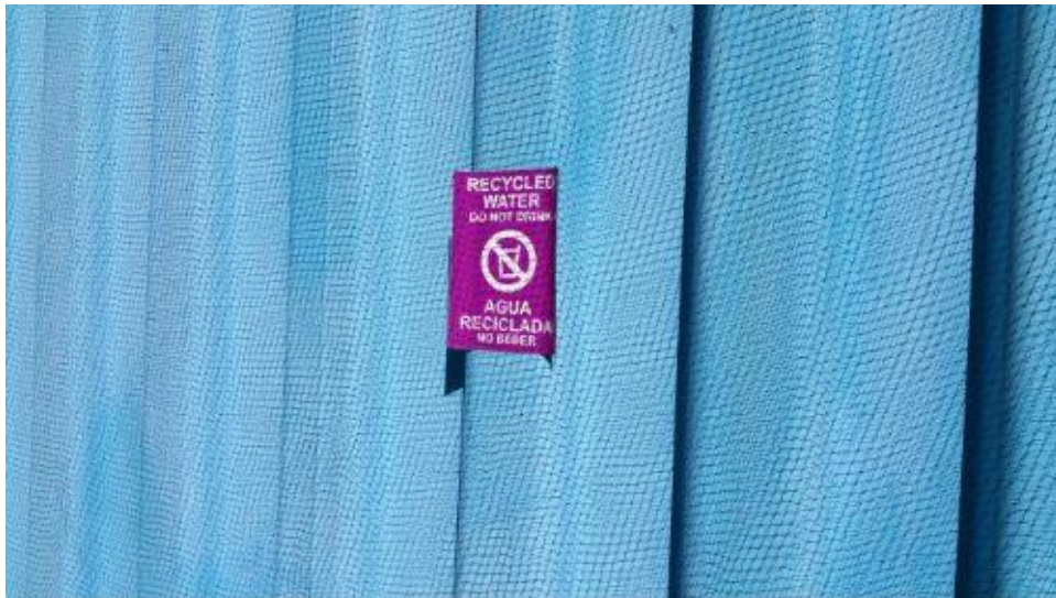
Caption Labelling on recycled water tanks.
