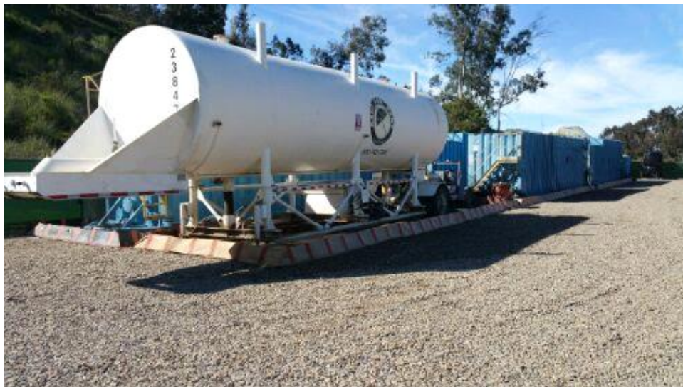
Caption Secondary containment around water pumps at Driving Range Yard.
