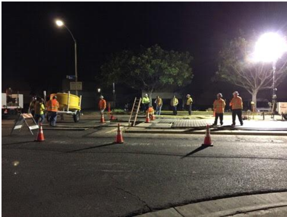
Caption Trenching activity with lighting and signage and traffic flaggers in place.
