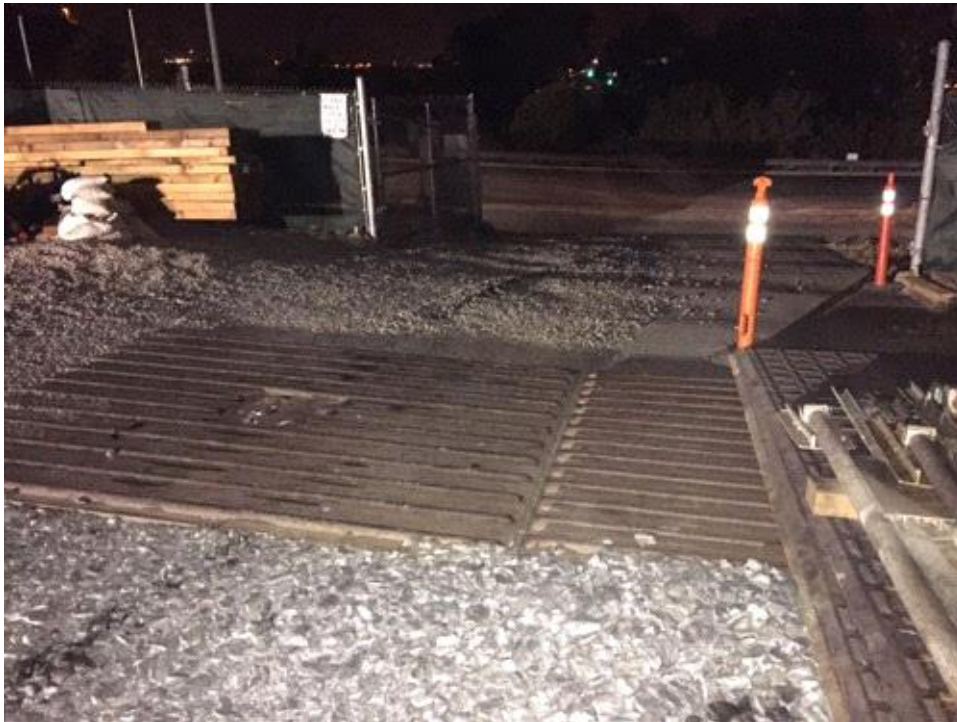
Caption Shaker plates in place at storage yard entrance. Photo Attributes Capture Date/Time: Wed Apr 26 2017 04:38:50 GMT-0700 (PDT) Coordinates: 32.891168, -117.191656 View Direction: West
