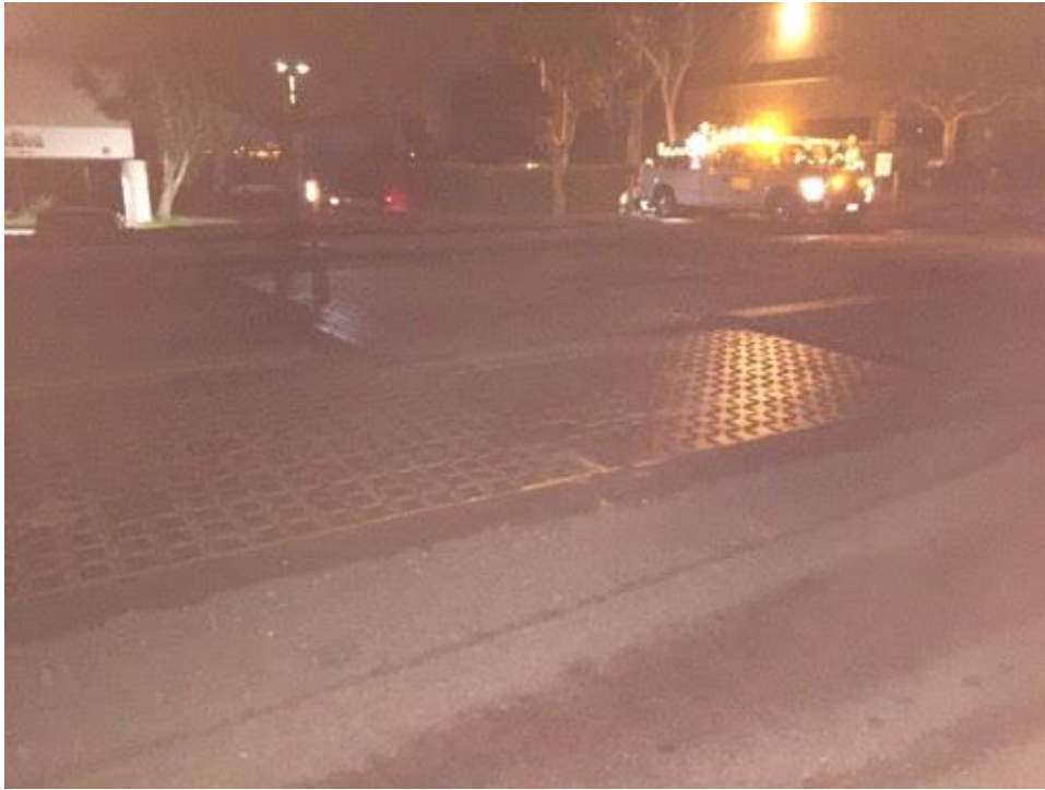
Caption Trenches put in place and sealed with asphalt upon completion of the night's work.
