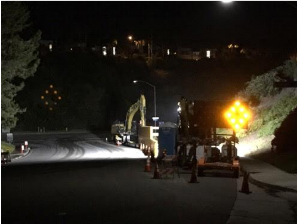
Caption Digital construction warning signage in place. Photo Attributes Capture Date/Time: Wed Apr 26 2017 05:08:41 GMT-0700 (PDT) Coordinates: 32.889451, -117.179914 View Direction: Southwest
