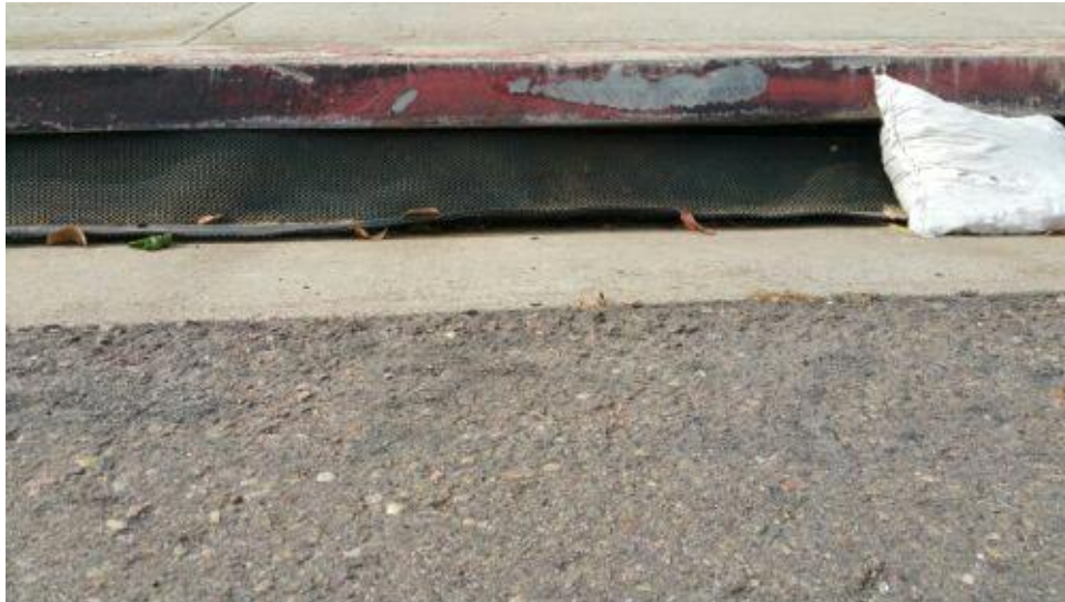
Caption Filter fabric not flush with road surface; Trade PI & Dunbrook.
