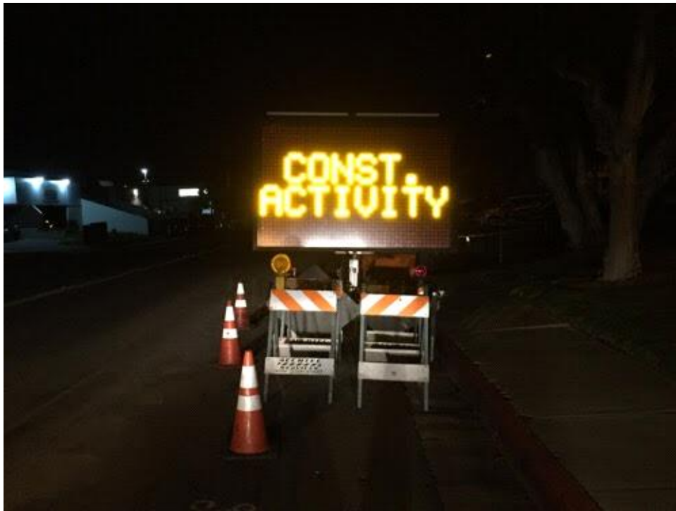
Caption Digital traffic signage in place.
