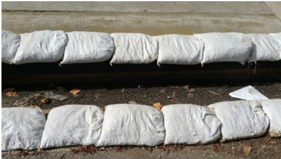
Caption Sediment caught by filter fabric, Trade St. staging area.
