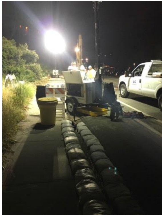
Caption Monitors and site tailboard just completed prior to lifting plates (Carrol Way). Notice BMPs installed at storm drain.
