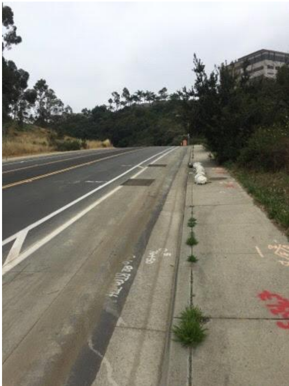
Caption Storm drain without water quality protection measures.
