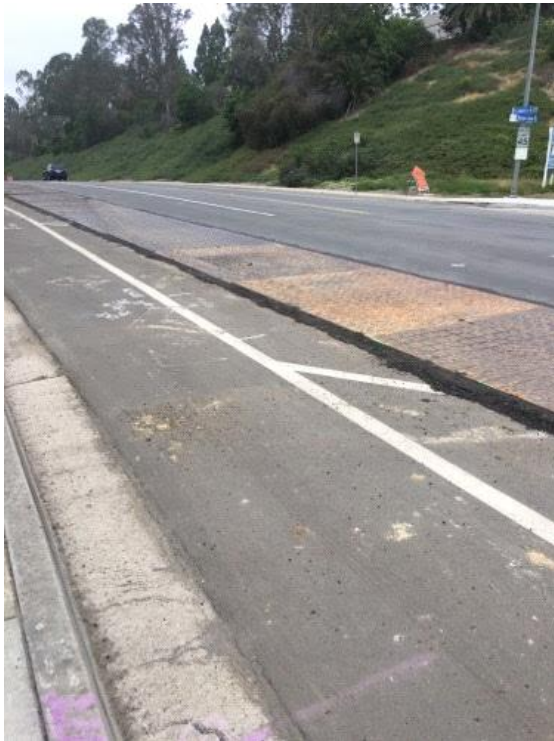
Caption Carrol Rd, note loose dirt and gravel
