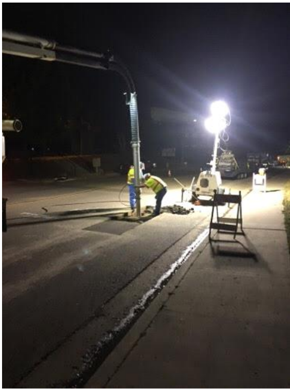
Caption Potholing on Trade Place
