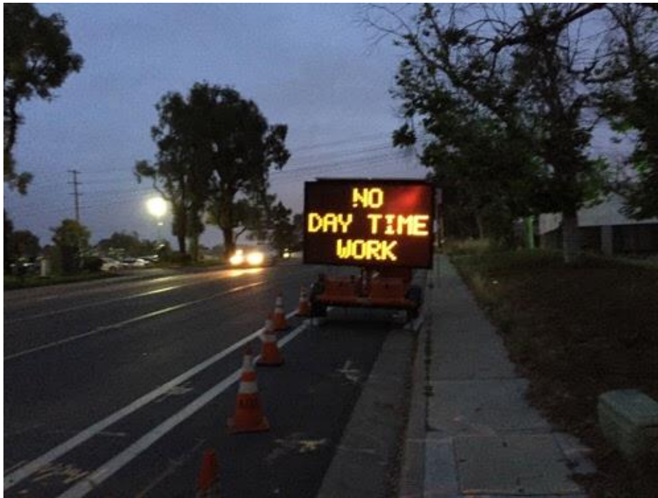
Caption Digital signage in place.
