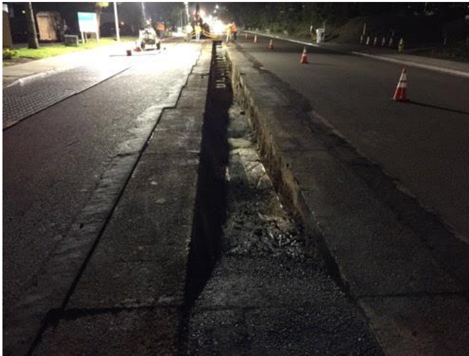
Caption Ramps installed in trenches for egress. Photo Attributes Capture Date/Time: Mon May 08 2017 21:32:54 GMT-0700 (PDT) Coordinates: 32.888779, -117.164341 View Direction: Northeast
