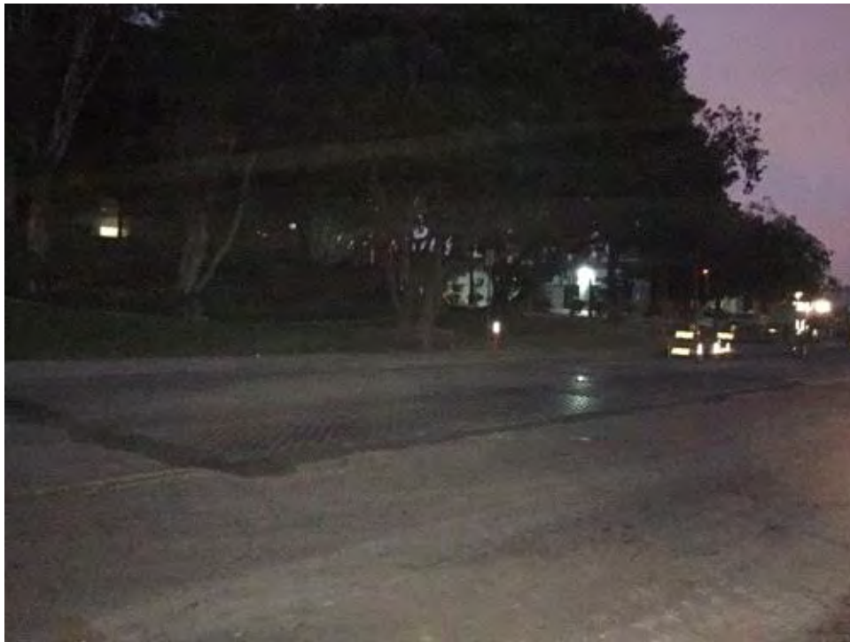
Caption Vault covered with steel plates and street returned to full public use.
