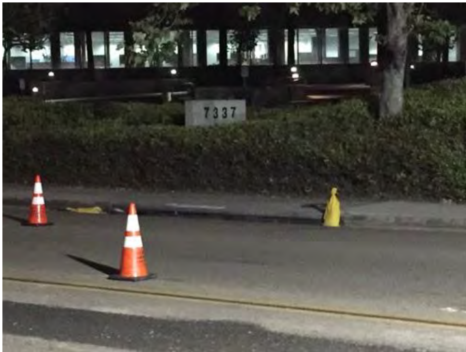
Caption BMPs in place and good working order.
