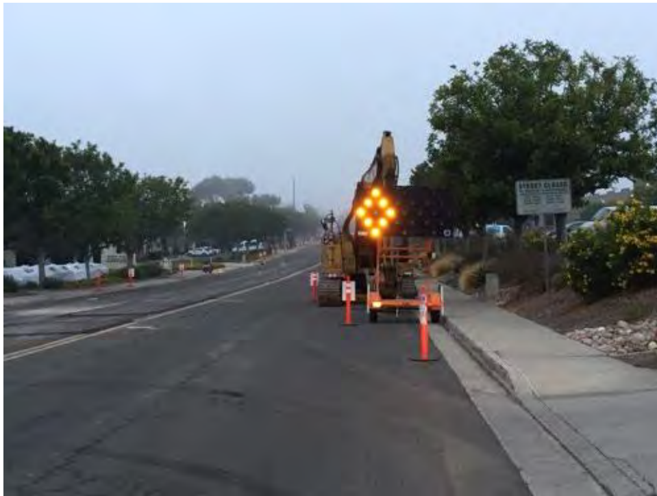
Caption Digital signage in place.
