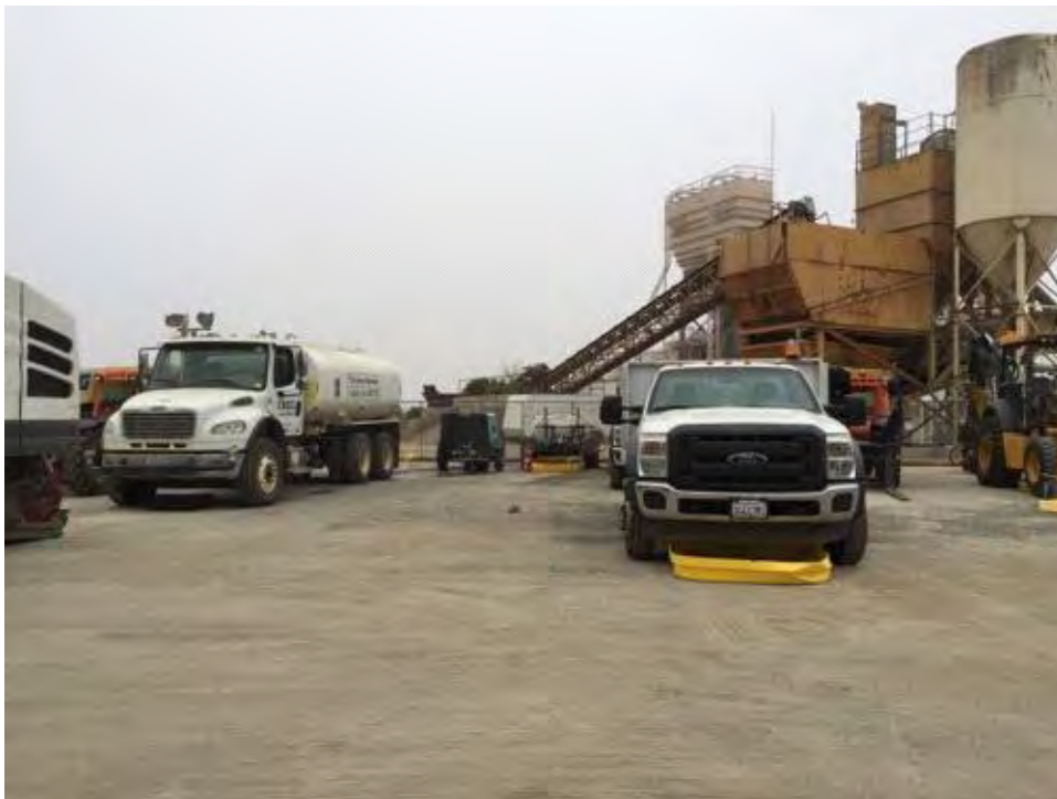
Caption Drip pans in place at Vulcan Staging Yard.
