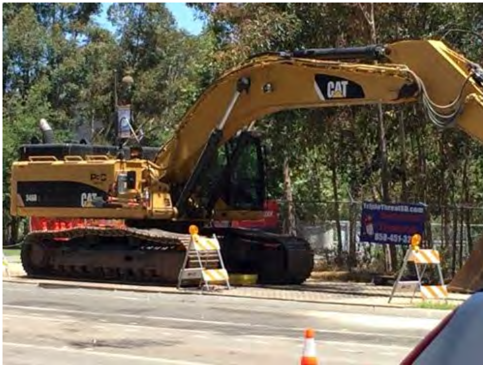
Caption Drip pan in place for excavator on Pomerado Road and Willow Creek Road.
