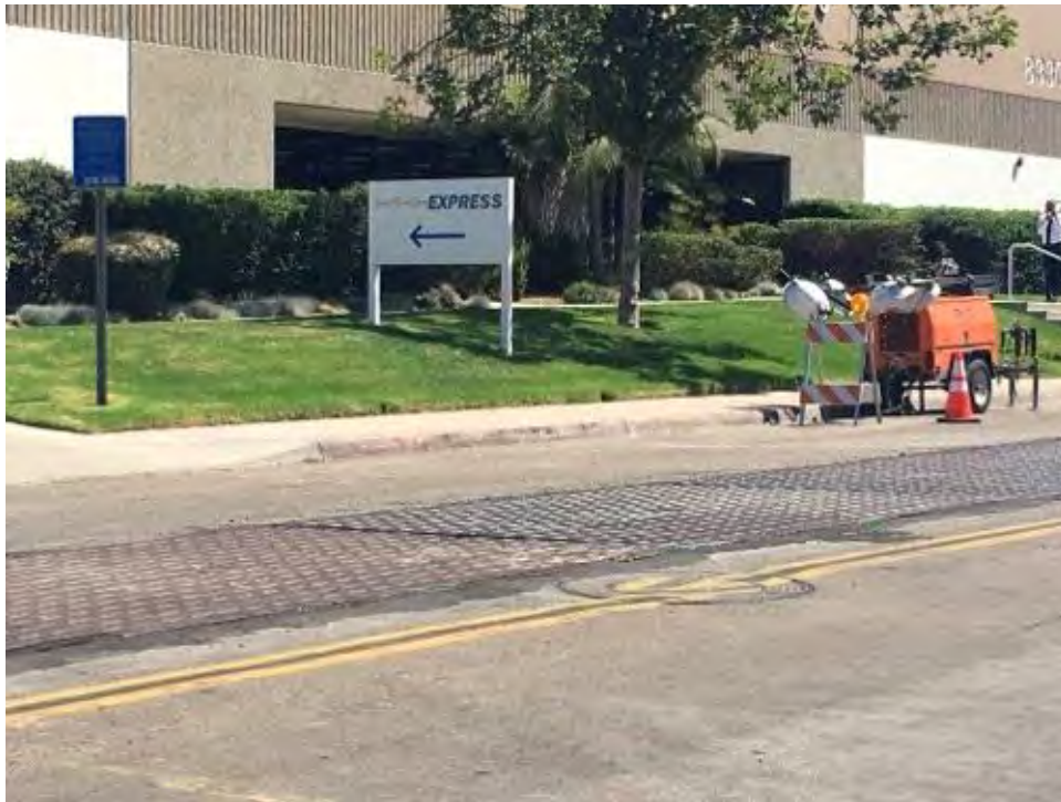
Caption Coldpatch asphalt debris on Miralani Drive.
