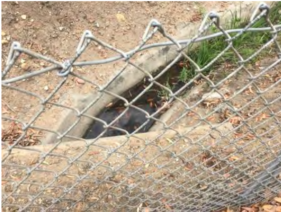
Caption Ponding offsite following morning rainstorm. Photo Attributes Capture Date/Time: Mon Jul 24 2017 15:34:03 GMT-0700 (PDT) Coordinates: 33.157055, -117.312533 View Direction: North
