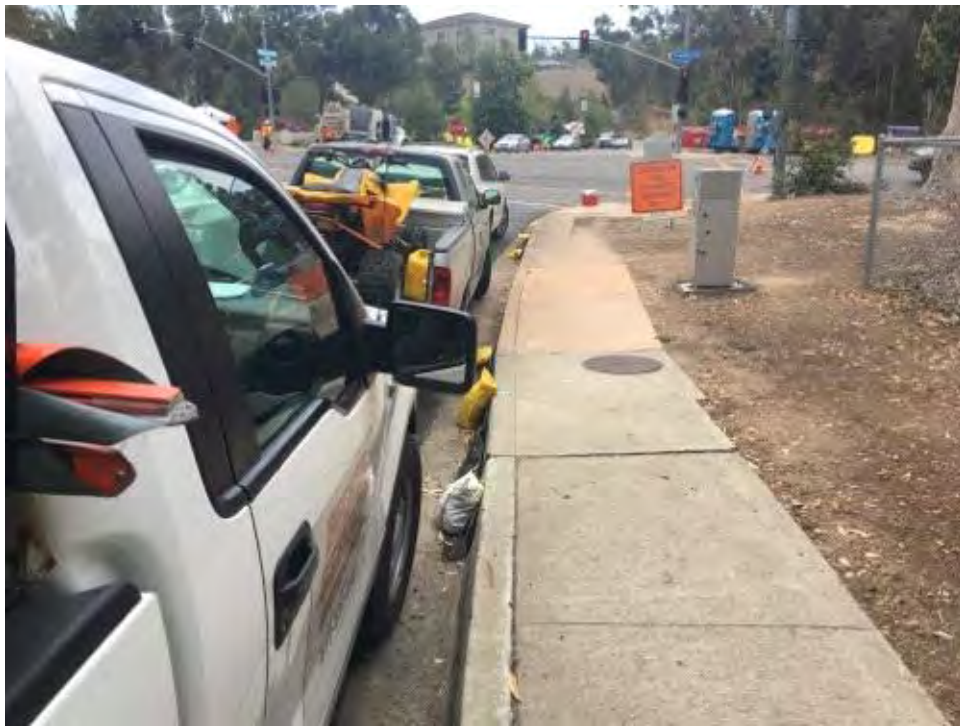
Caption Pomerado Road/Avenue of Nations BMPs functioning following morning rainstorm.
