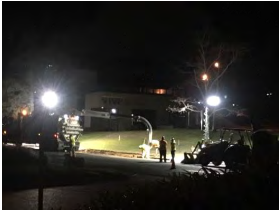
Caption Potholing/excavation on Activity Road. Photo Attributes Capture Date/Time: Wed Jul 26 2017 23:06:54 GMT-0700 (PDT) Coordinates: 32.896514, -117.134524 View Direction: Southeast
