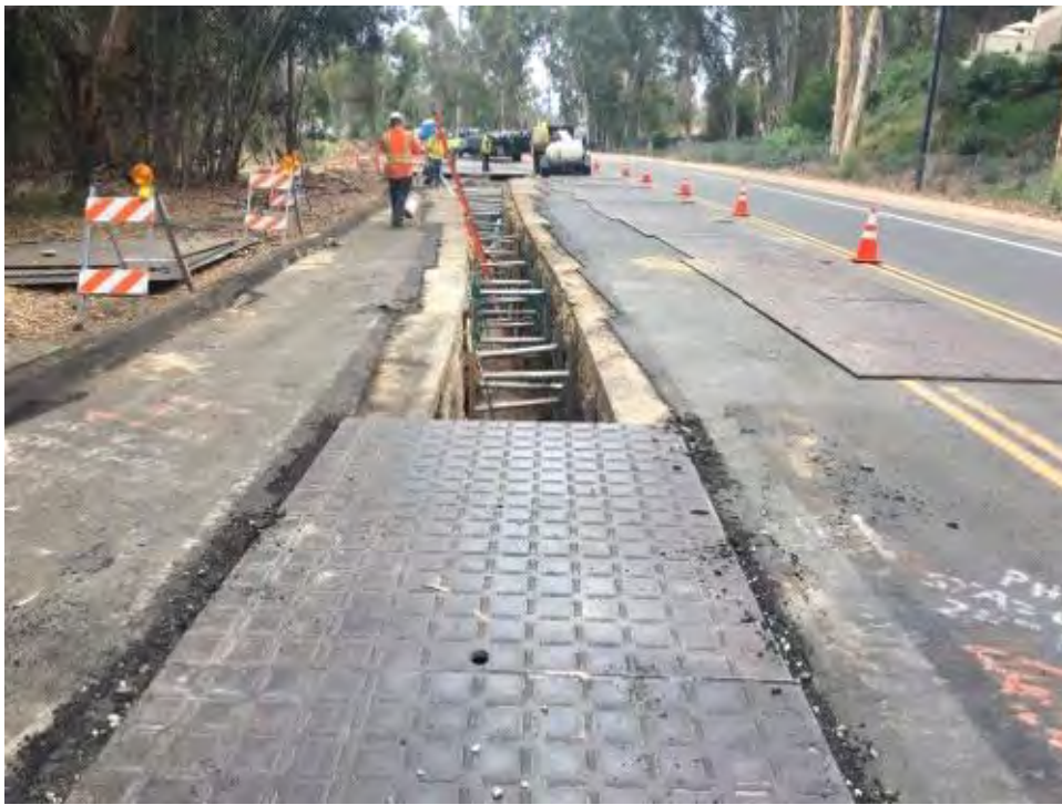
Caption Trench along Pomerado Road Photo Attributes Capture Date/Time: Mon Jul 24 2017 15:34:43 GMT-0700 (PDT) Coordinates: 33.157055, -117.312533 View Direction: West
