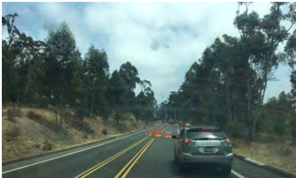
Caption Traffic control on Pomerado Road just west of active vault work site.
