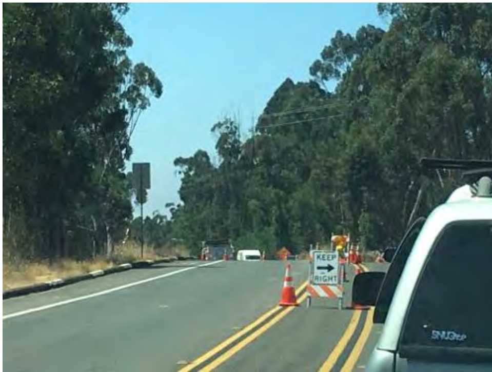
Caption Traffic control on Pomerado Road going west, east of active work site.
