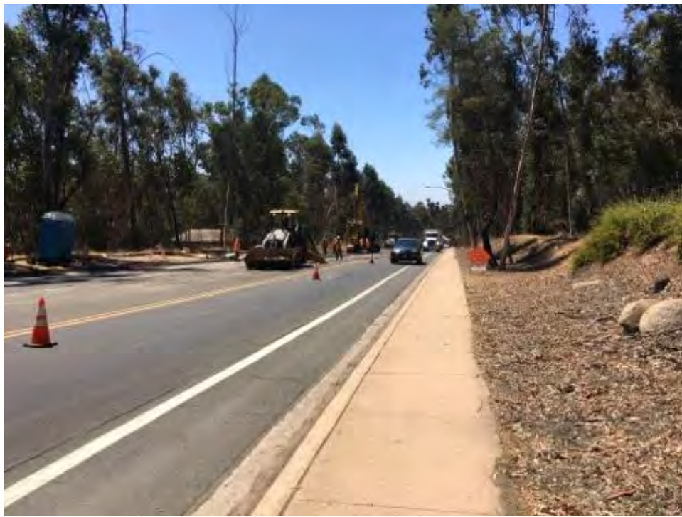
Caption Active work site on Pomerado Road east of Avenue of Nations and West of Scripps Ranch Blvd.
