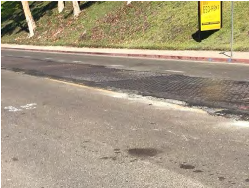
Caption Abundant asphalt debris along western portion of Trade Street.
