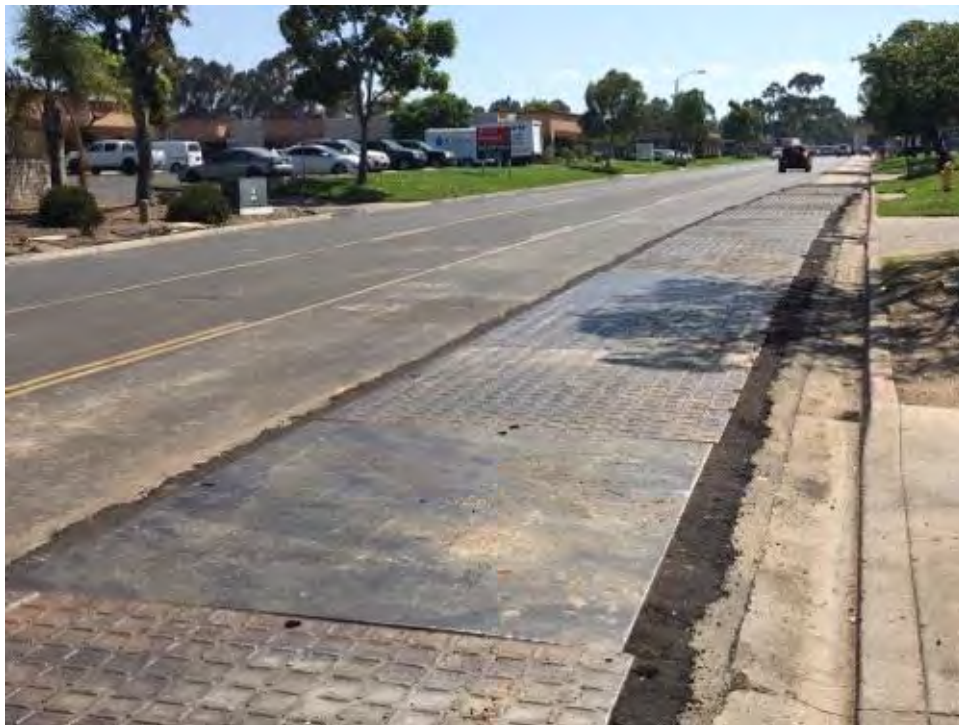
Caption Abundant asphalt debris on Activity Road.
