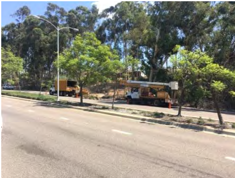
Caption Unrelated tree trimming near intersection of Scripps Ranch Blvd and Pomerado Road.
