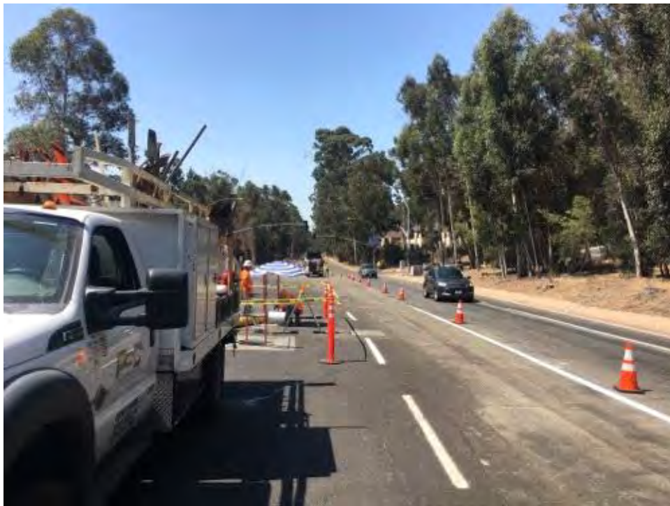
Caption Vault and traffic control just west of Ave of Nations.
