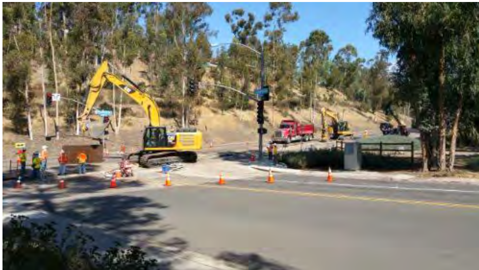
Caption Trenching on Pomerado Road and Fairbrook Drive. Monitors and fire equipment on hand.
