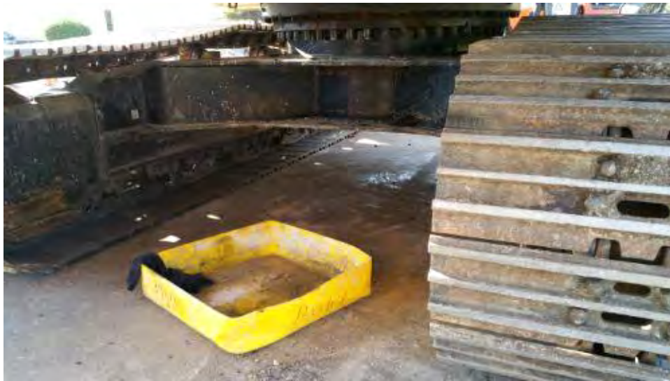
Caption Drip pans are placed beneath equipment, but not actually beneath those that would leak oil, making them ineffective. Padgett Road storage area. No leaks present.
