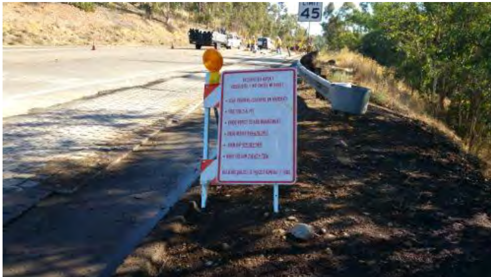
Caption Restricted site signage along Pomerado Road at Avenida Magnifica. Trenching in background.
