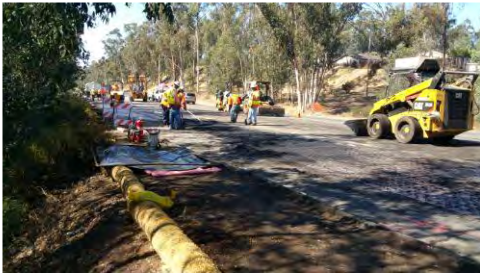
Caption Fire safety tools on hand, Pomerado Road and Avenida Magnifica.
