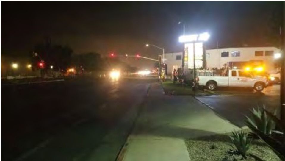
Caption Flashing stop lights only visible traffic control at Black Mtn Road & Miramar. Traffic flows into single right and left lanes; flaggers direct traffic through work area.
