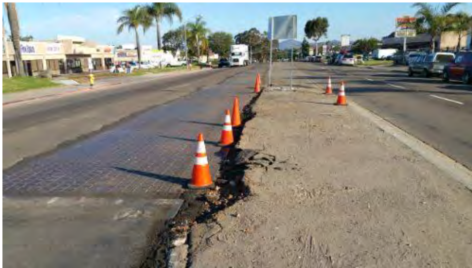
Caption Cones placed next to broken traffic island, Black Mtn. Road.
