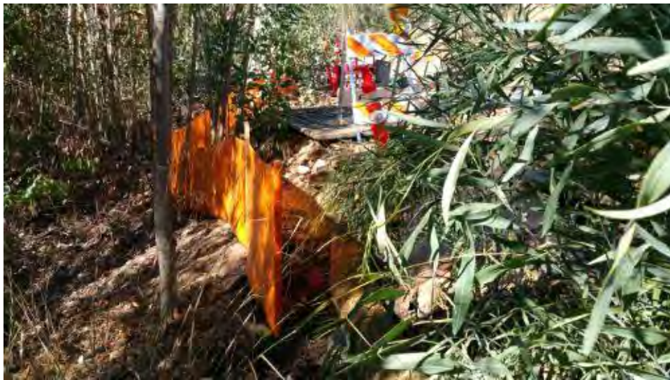
Caption Silt fencing behind straw wattles adjacent to small storage area off Pomerado Road.
