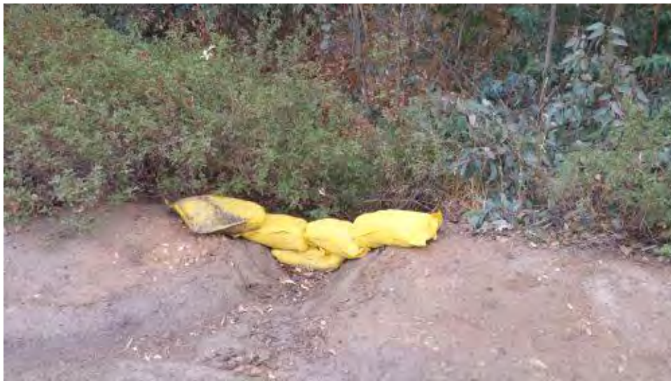
Caption Gravel bag BMP enhanced and fully functional on Pomerado Road east of Avenida Magnifica. (Noted in previous report).
