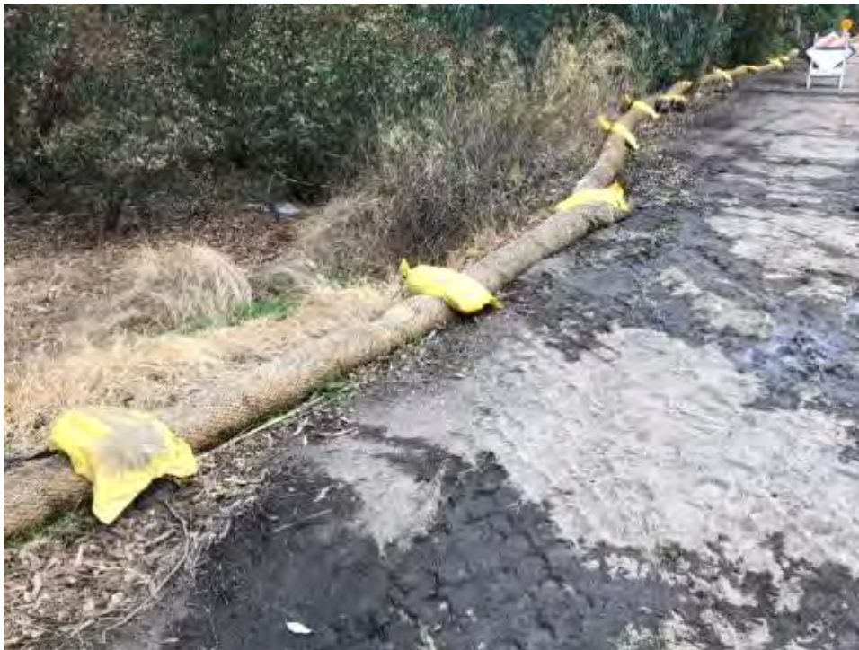
Caption BMPs improperly installed all along disturbed area at section 535+50 along Pomerado Road.
