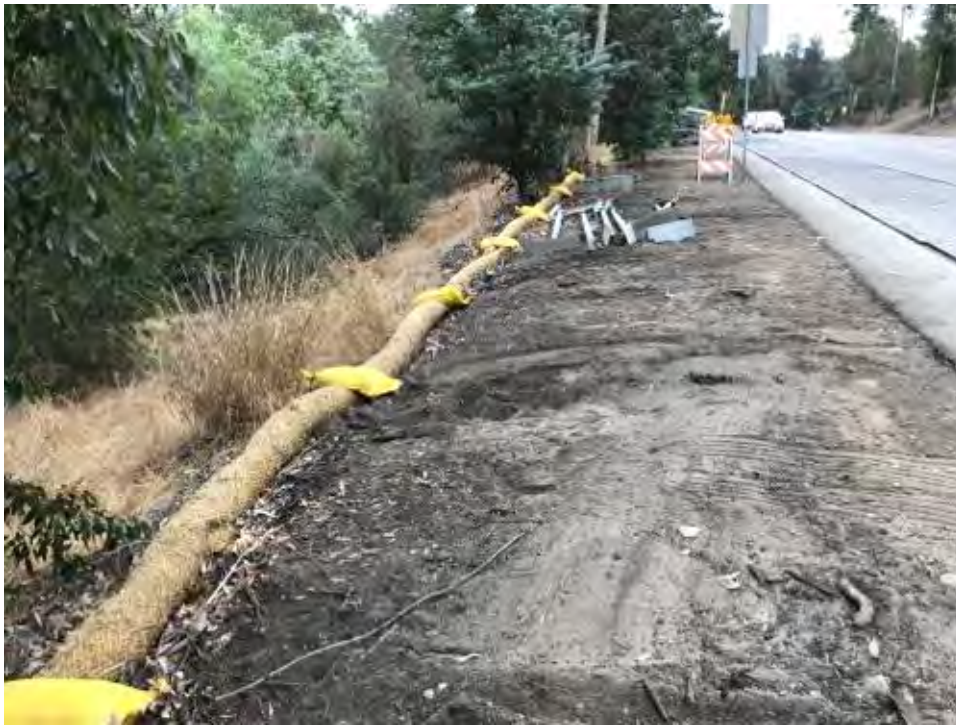
Caption BMPs improperly installed at section 551+00 along disturbed area on Pomerado Road east of Fairbrook Road.
