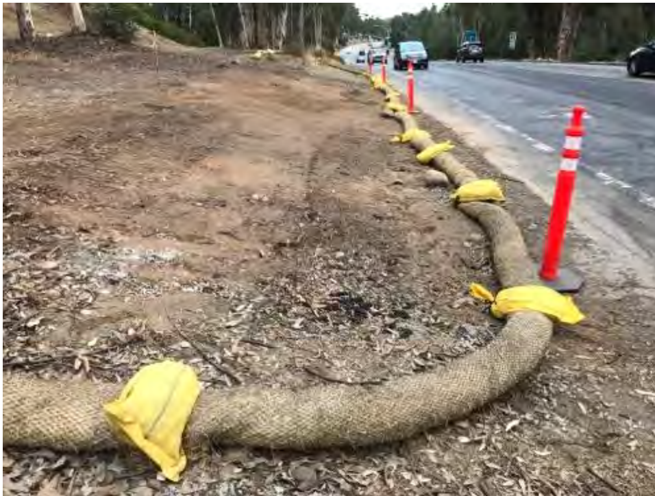
Caption BMPs at section 507+25 on Pomerado Road are improperly installed.
