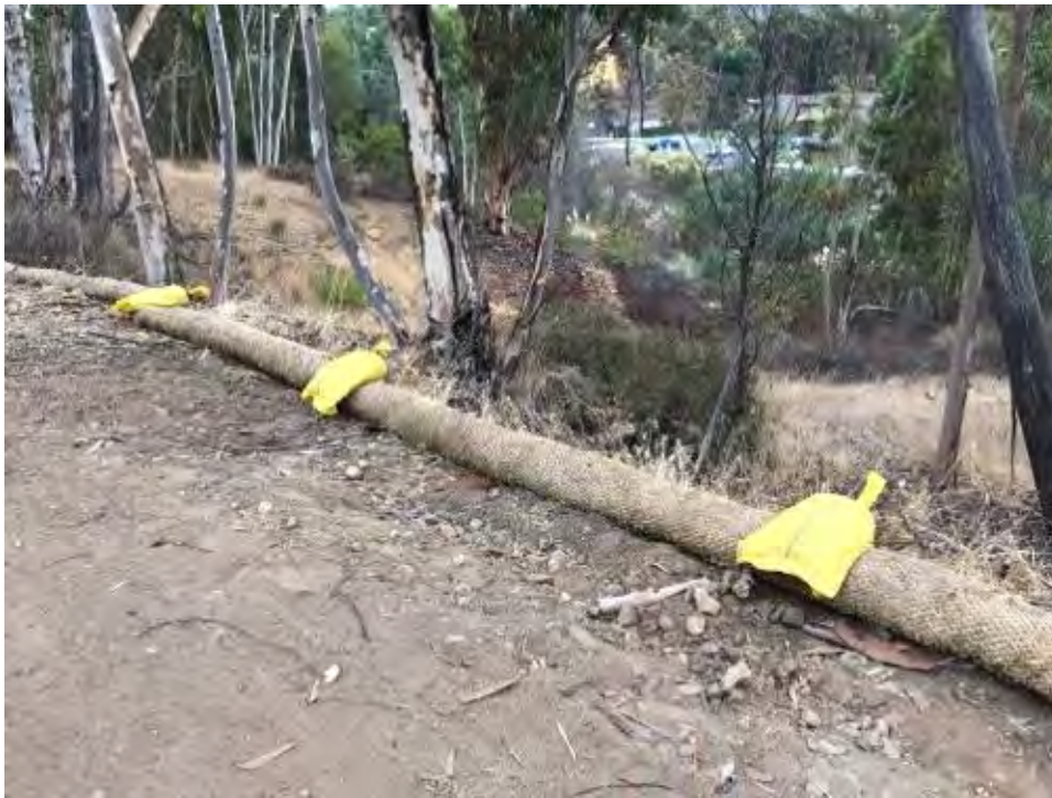
Caption BMPs at section 485+25 on Pomerado Road improperly installed Will not protect drainage basin.
