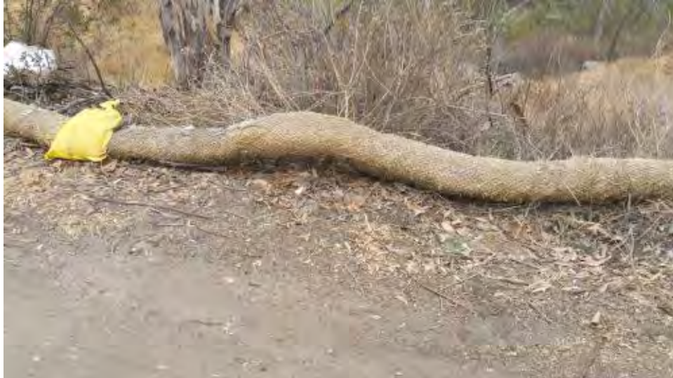
Caption Improper erosion control BMP installation on Pomerado Road.
