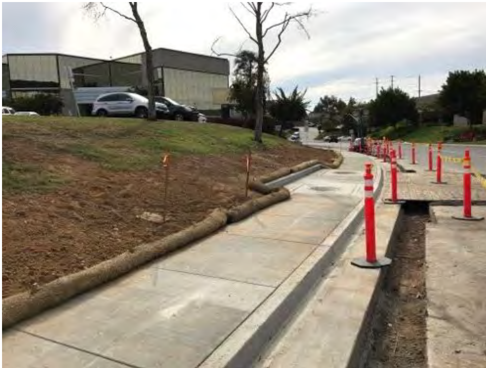
Caption BMPs still need to be trenched in place on Activity Road.
