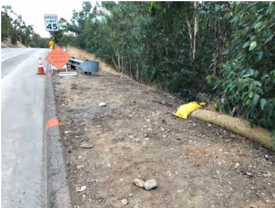
Caption BMPs missing at section 517 + 50 on Pomerado Road east of Avenida Magnifica.
