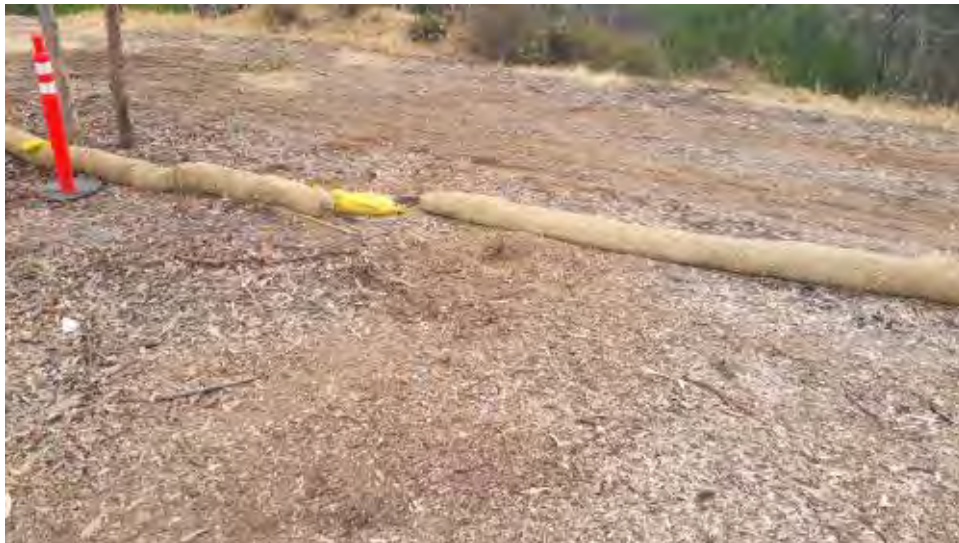
Caption Improper placement of erosion control BMPs on Pomerado Road east of Avenida Magnifica.
