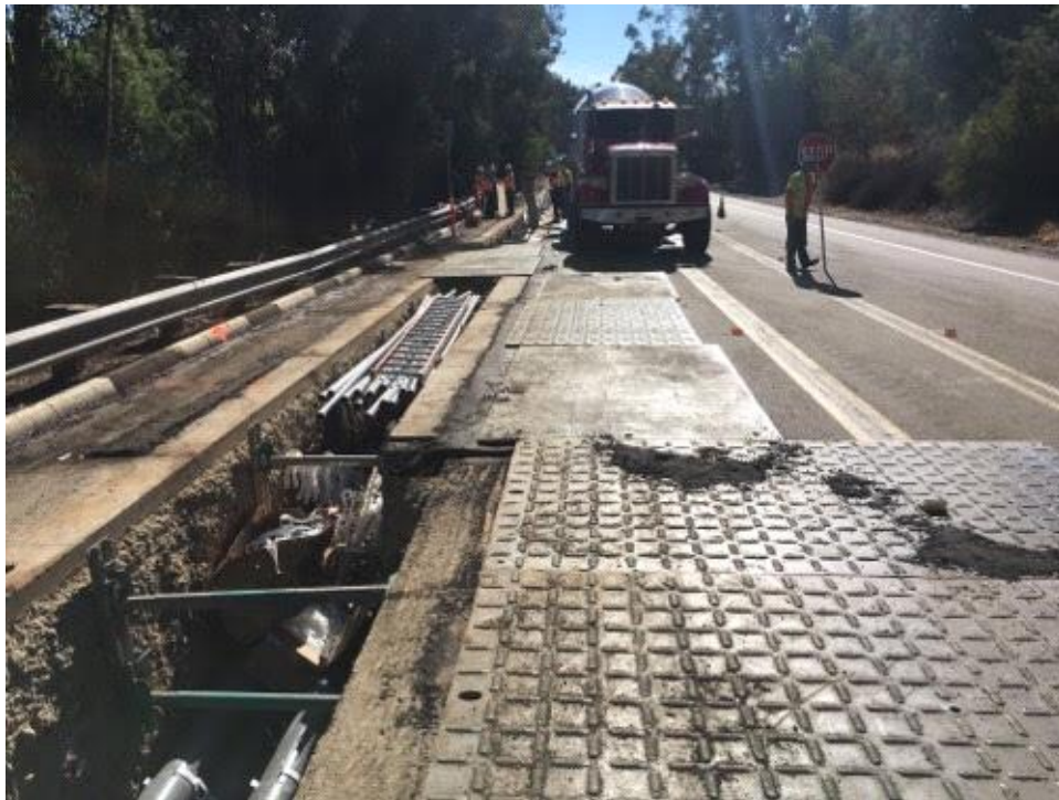
Caption Trench and concrete work on Pomerado Road west of Semillon Blvd.
