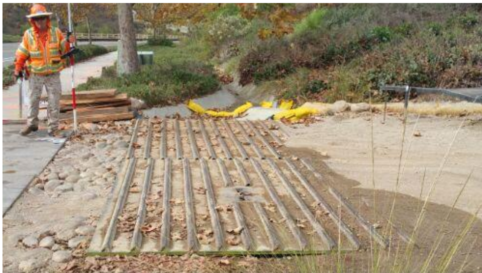
Caption Rumble plates and gravel bags installed on road to pole sites.
