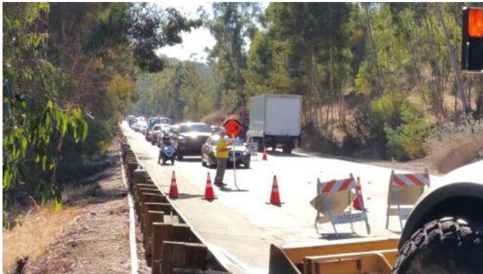
Caption Traffic control at west end of main work area on Pomerado Road.
