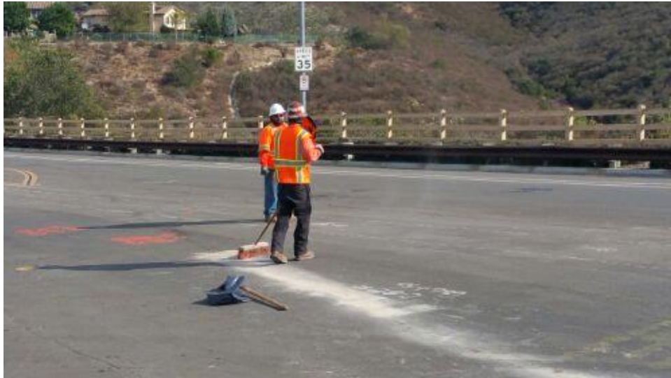
Caption Cleaned-up fuel spill site at Stonebridge Parkway and Rose Garden.
