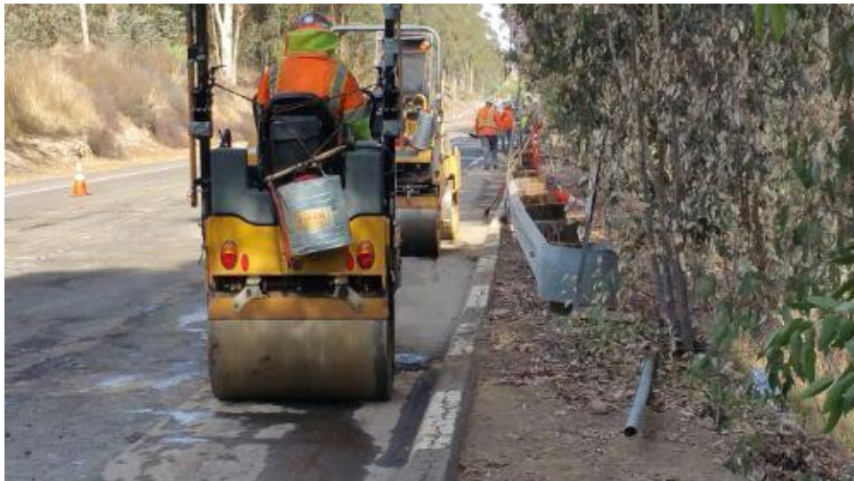
Caption Fire control gear on vehicles and available at paving crew work site on Pomerado Road.
