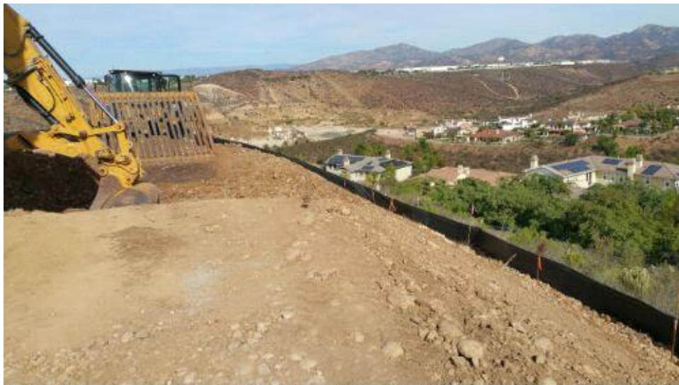
Caption Excavation for retaining wall at PO5. Photo Attributes Capture Date/Time: Tue Nov 28 2017 12:12:18 GMT-0800 (PST) Coordinates: 32.922523, -117.042395 View Direction: North
