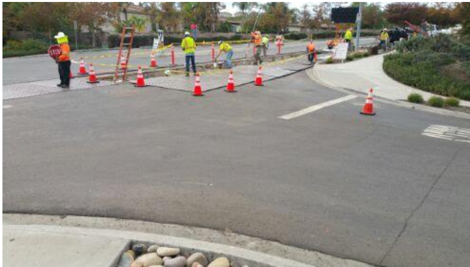
Caption Active work area on Stonebridge Parkway set up to allow access to Brookside Lane.
