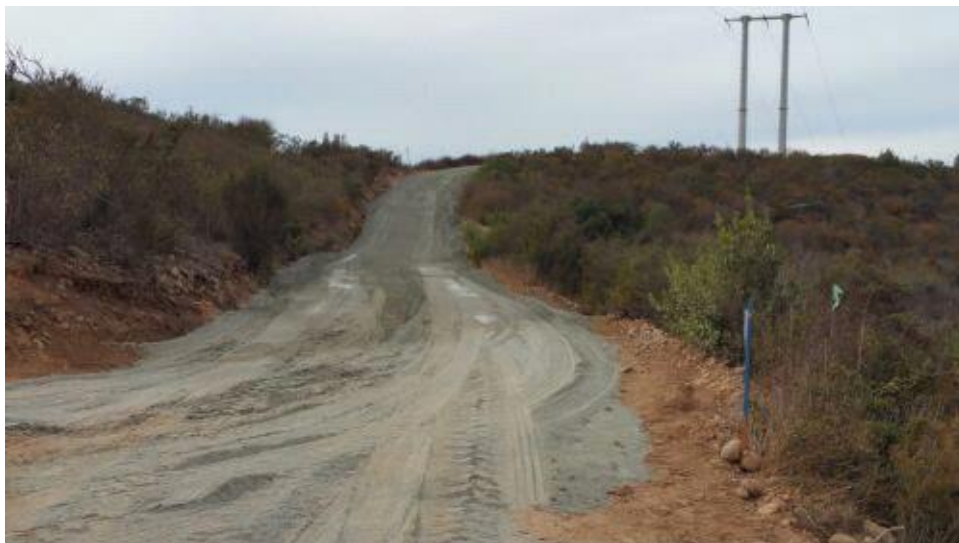
Caption Fill material for PO5 spread out on upper access road still to be watered.
