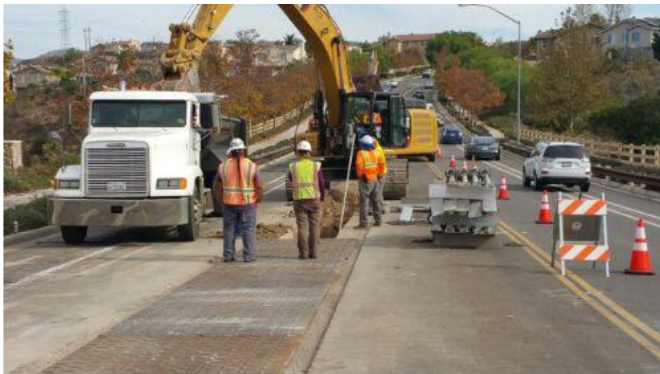
Caption Excavation in Stonebridge Parkway, 2 monitors present. Photo Attributes Capture Date/Time: Tue Nov 28 2017 11:32:46 GMT-0800 (PST)
