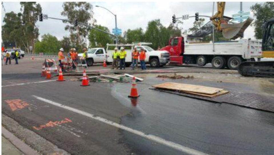
Caption Broken water line with City crew working on repair.
