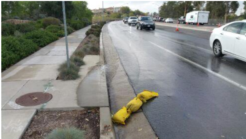
Caption Water flow was directed into storm drain system during busted water line emergency.
