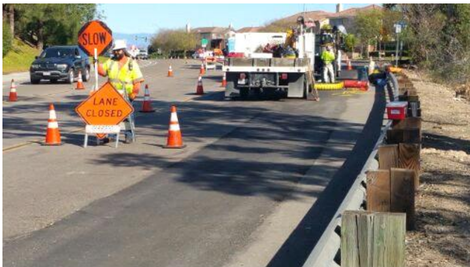
Caption Approach to work zone from west (Pomerado Road). Mandreling in background.
