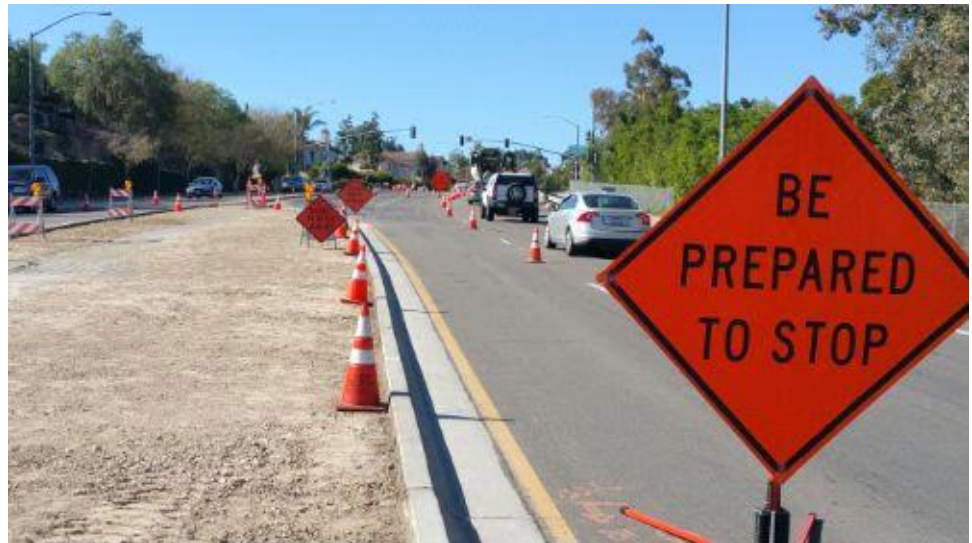
Caption Four warning signs approaching corner of Pomerado Road.
