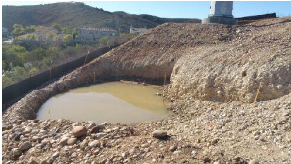
Caption Excavated area around base of PO5 is holding water.
