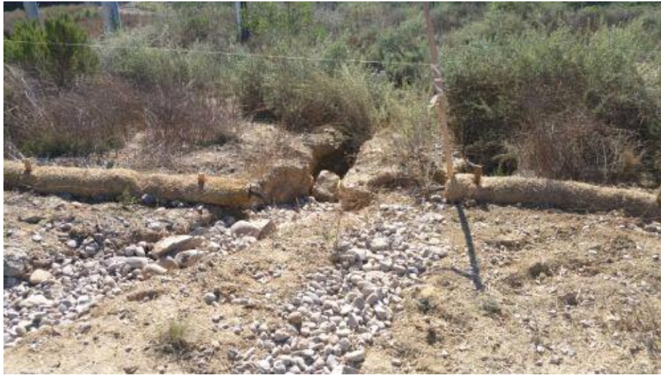
Caption Gap in straw wattles is to allow water from outflow pipe at CC MM CP to flow across work site and downslope, per LEI.
