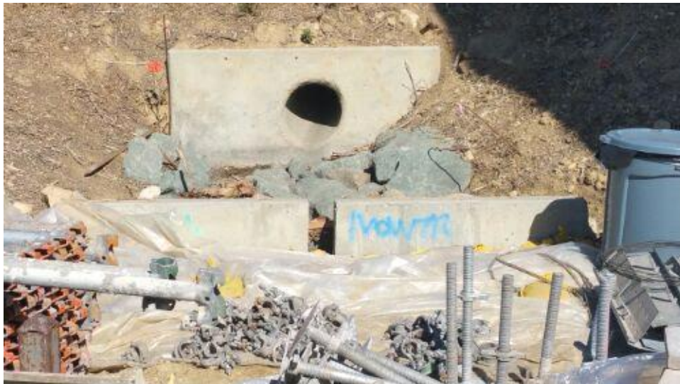
Caption Erosion control below outfall onto CC MM CP.
