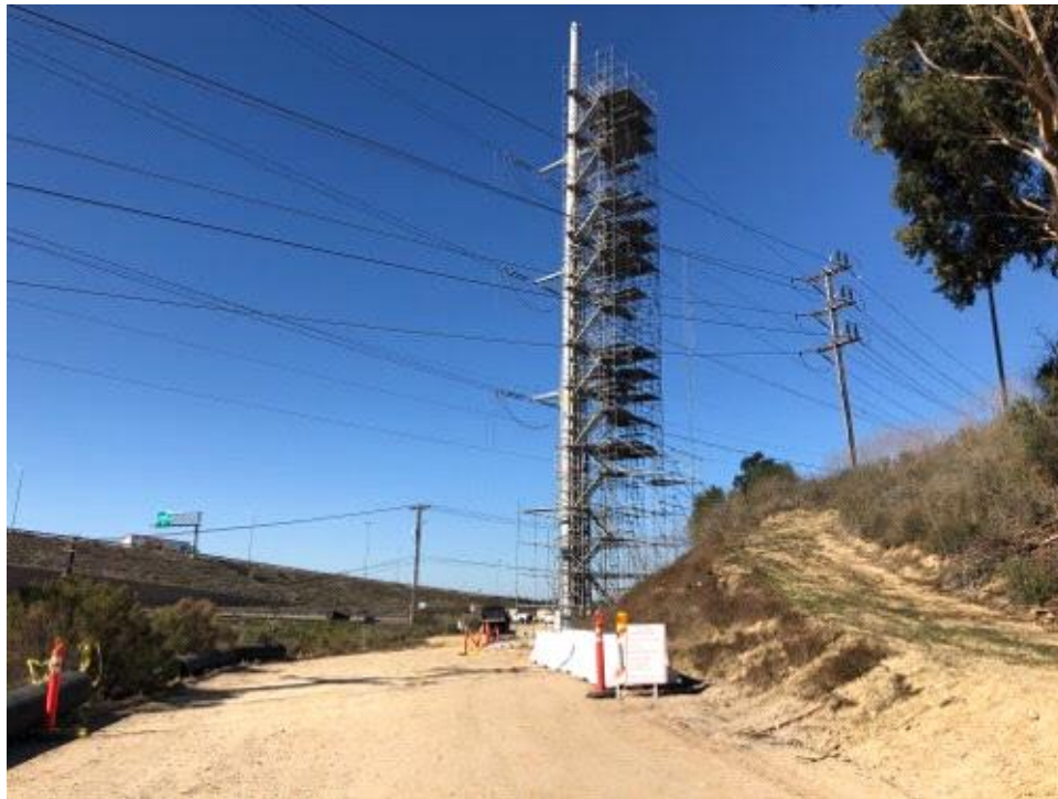
Caption CCM MCP pole and scaffolding.
