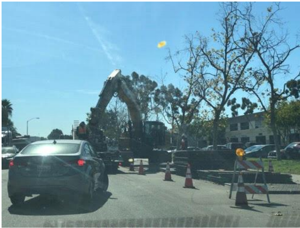
Caption Street plate storage, active traffic control in place on Padgett Street.
