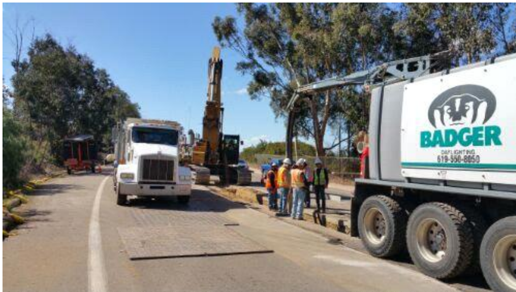
Caption Excavation on Pomerado Road. Cultural resources and Native American monitors on hand.
