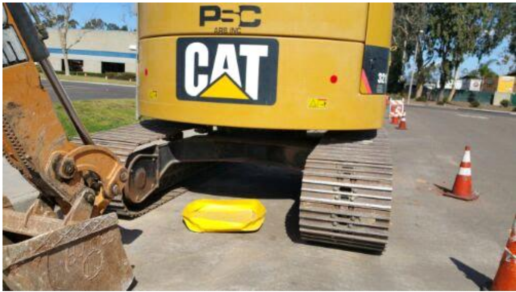
Caption Drip pan is not below point where a leak would occur for Cat 361036 at Padgett Road staging area.
