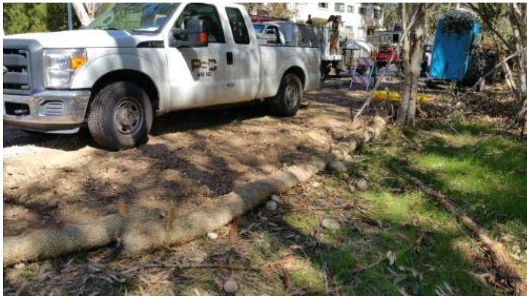
Caption Repaired straw wattles at station139+00 on Pomerado Road.
