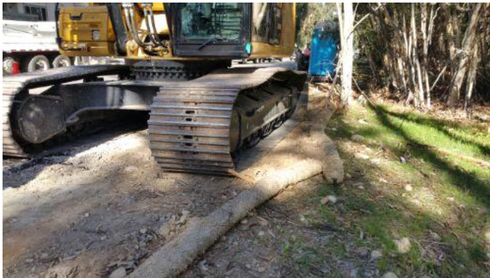
Caption Straw wattles damaged on Pomerado Road, about station 439+00.
