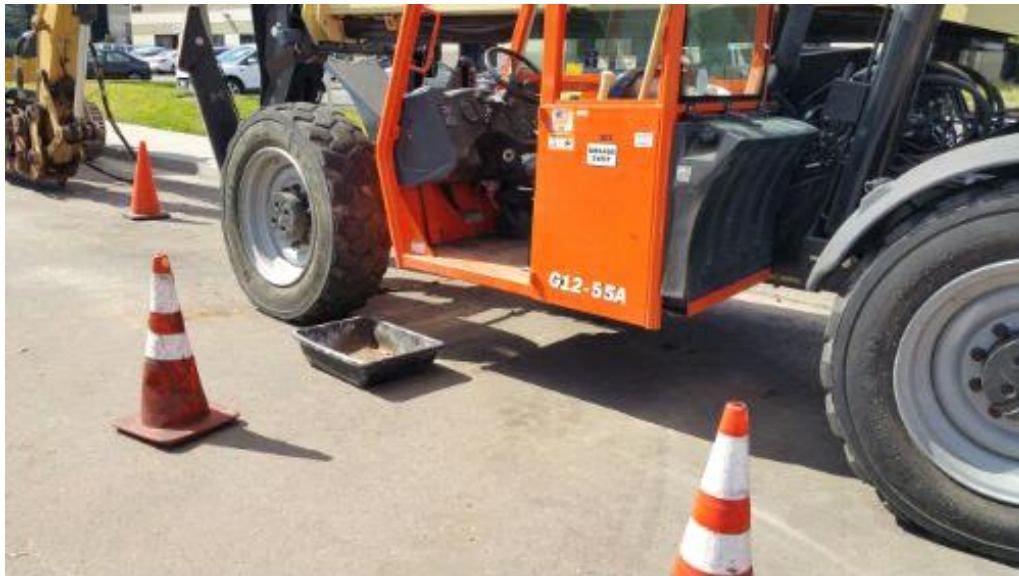
Caption Drip pan is not beneath equipment (265011) at Padgett Road staging area.
