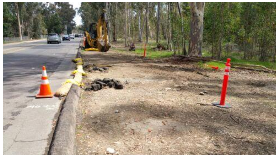
Caption Straw wattles put in place, MPR staging area on Pomerado Road.
