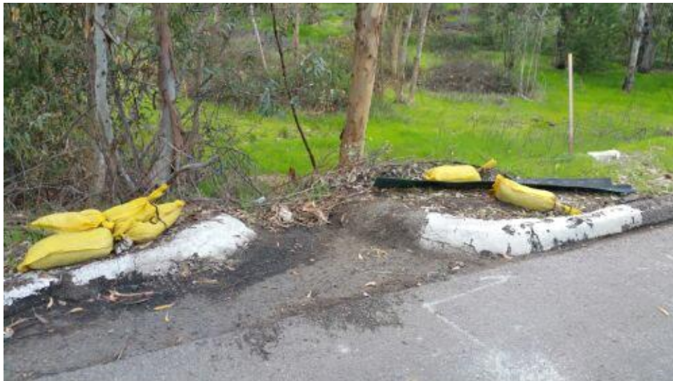
Caption Erosion control BMPs removed at Station 435+00: indicating point is not within active work area.
