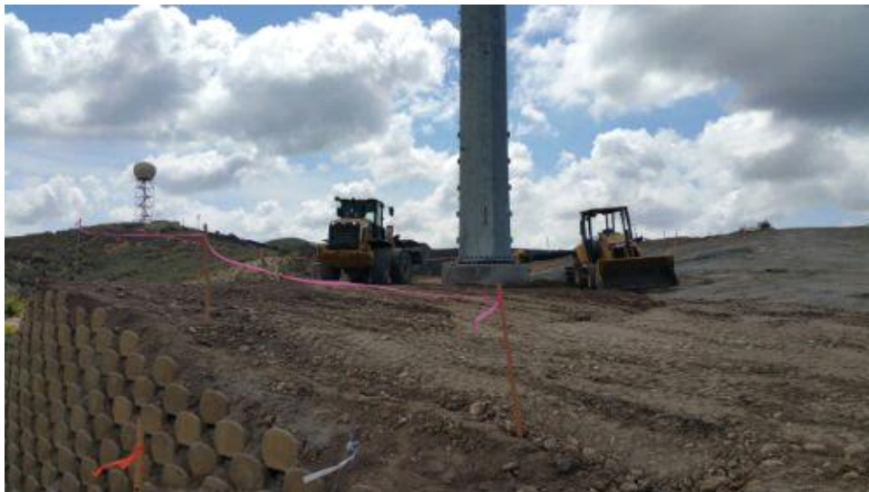
Caption Grading at PO5. Photo Attributes Capture Date/Time: Fri Mar 23 2018 13:08:56 GMT-0700 (PDT) Coordinates: 32.922769, -117.042329 View Direction: South
