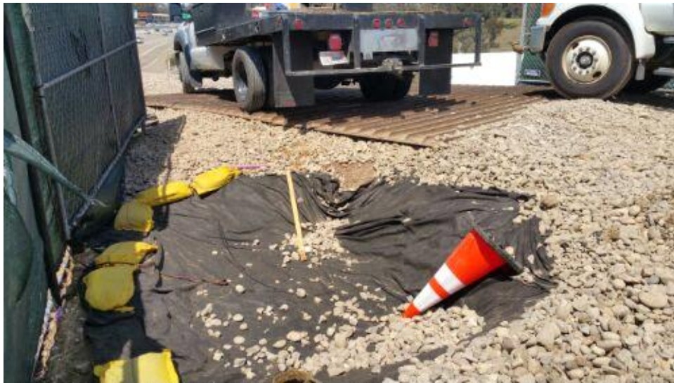
Caption Drain protection and rumble plates at east side I-15 sending pit work site.
