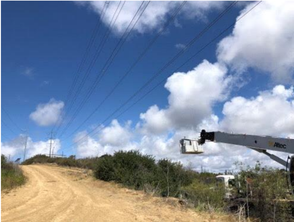
Caption Pull equipment north of CC MM CP and south of Lusk Boulevard.
