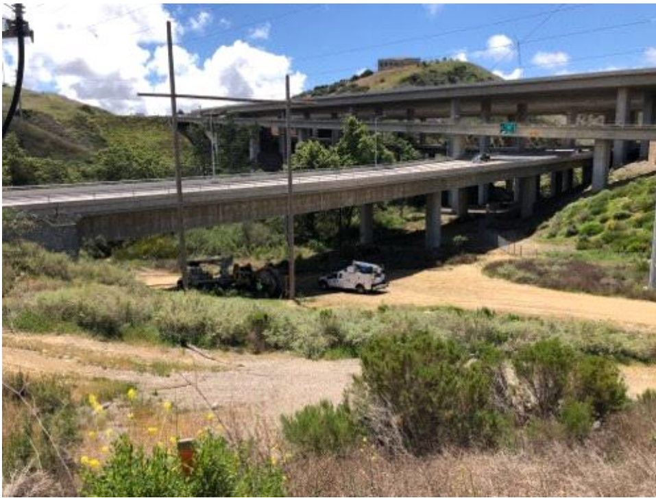
Caption Pull equipment (pulling wire under Carroll Canyon Road east of I-805.).
