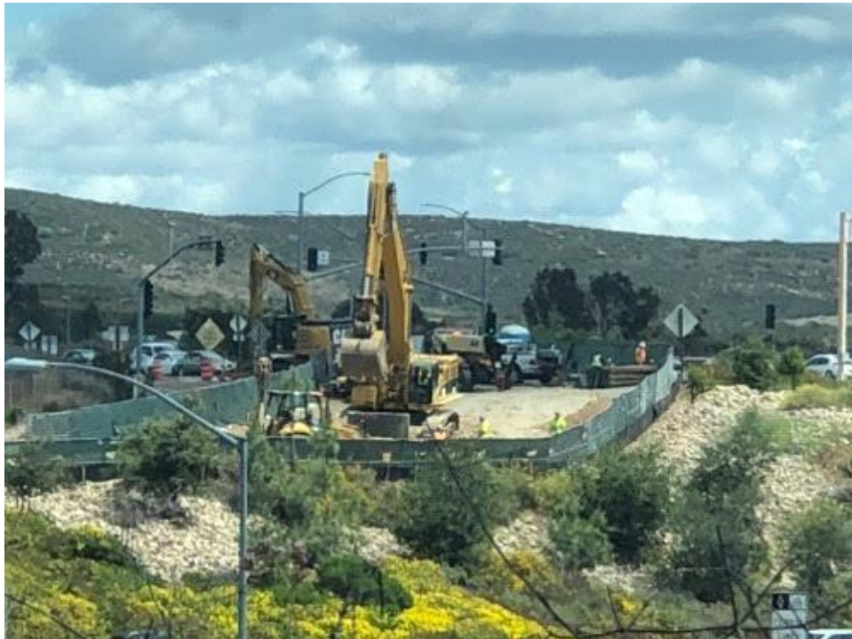
Caption Excavation at eastern bore pit location Photo Attributes Capture Date/Time: Thu Apr 19 2018 13:33:32 GMT-0700 (PDT) Coordinates: 32.894446, -117.117288 View Direction: East
