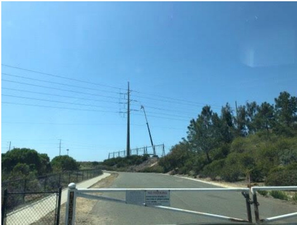
Caption Overhead crew near Penasquitos Substation.
