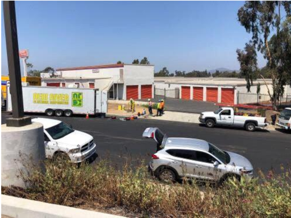
Caption Vault west of bore pit. Photo Attributes Capture Date/Time: Sat Aug 18 2018 12:48:54 GMT-0700 (PDT) Coordinates: 32.894653, -117.117715 View Direction: North
