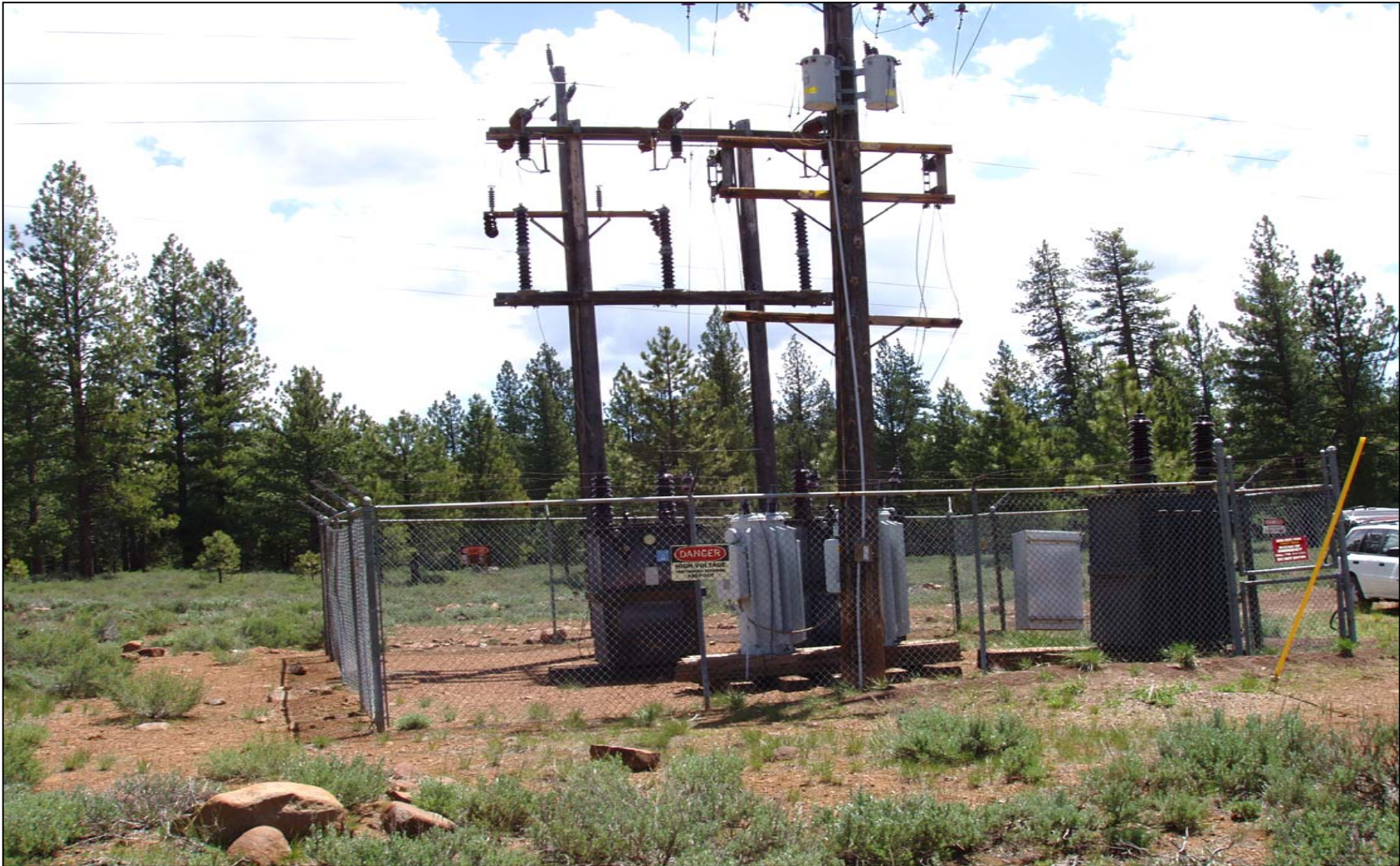
Photo 1: Existing Hobart Substation (looking east).
