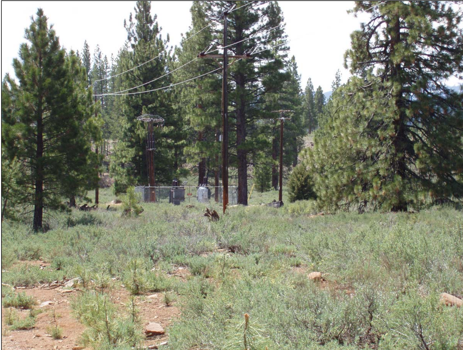
Photo 2: Existing Hobart Substation (looking south-west from private road)
