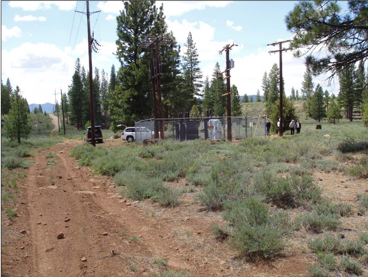
Photo 4.1-2: Existing substation, looking south from the access road.
