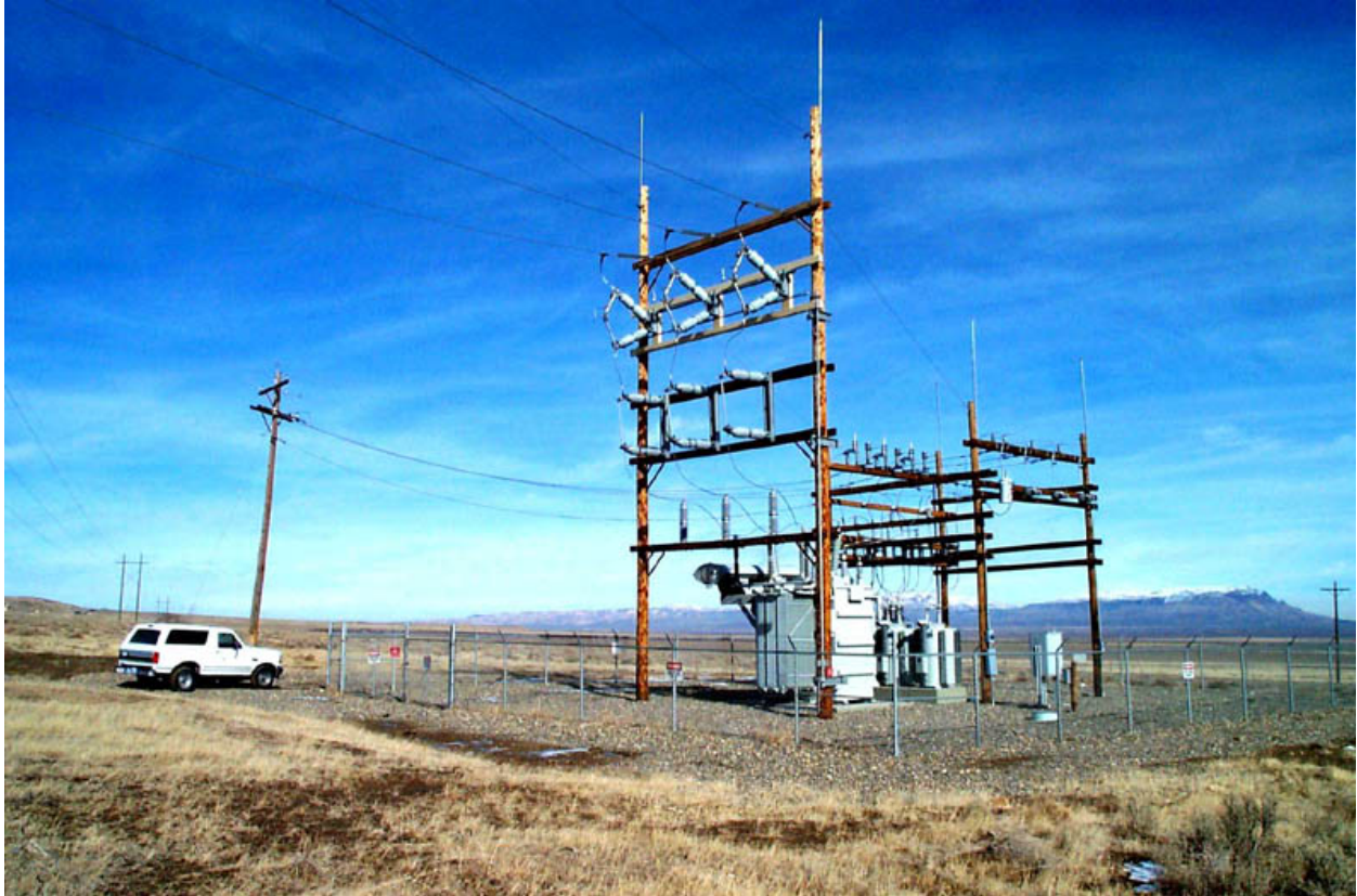
Osgood Substation, an example of the size and scope of the rebuild project.
