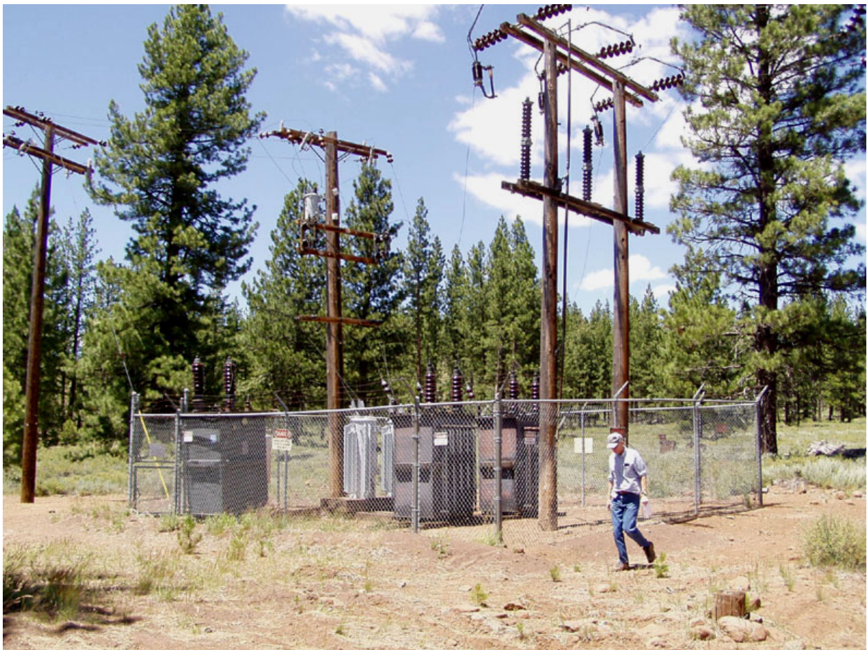
The existing Hobart Mills Substation.
