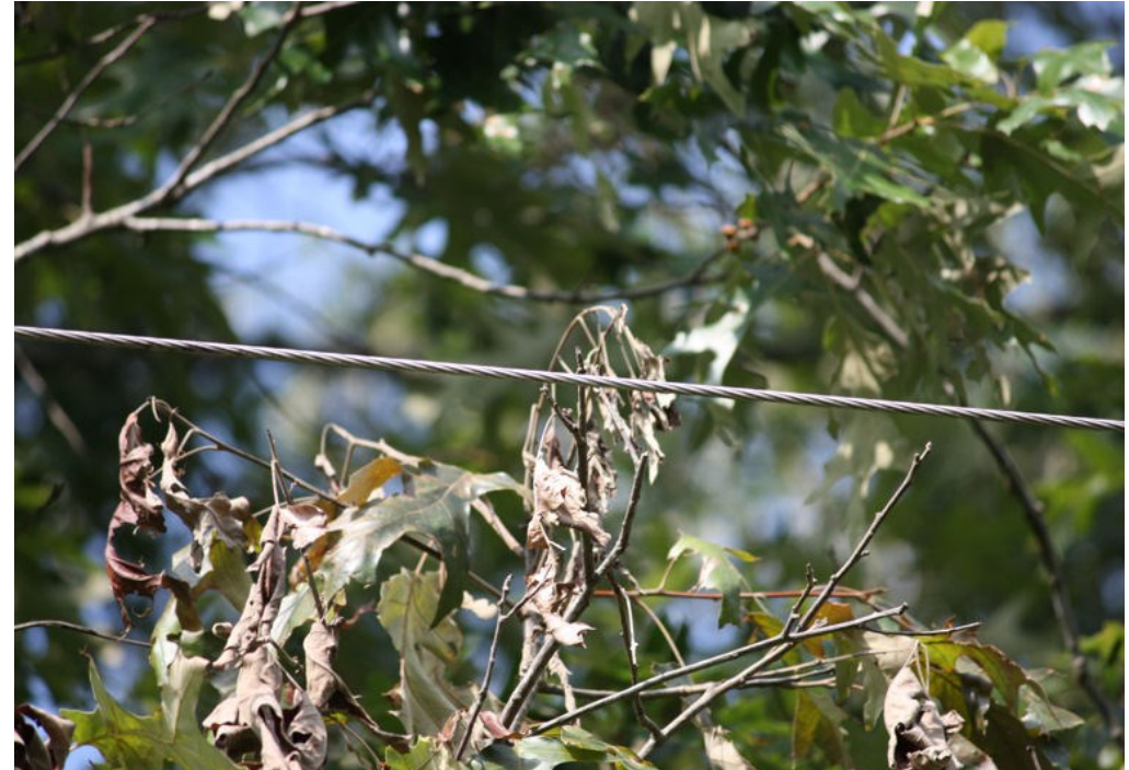
Vegetation fault Multiple flashovers in a 24-hour period Detected and corrected with DFA
