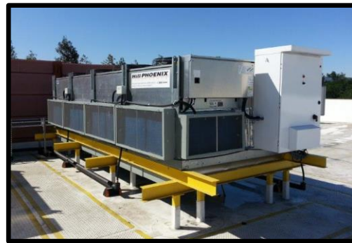
Example Refrigeration Condensing Unit
