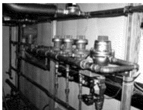
Figure 4: Flow Control Valve Array and Mass Flow Meter
