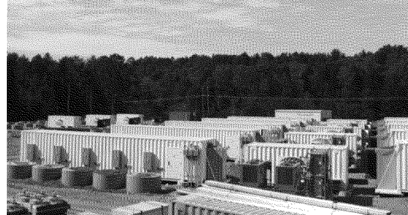
20 MW, Stephentown, MA
